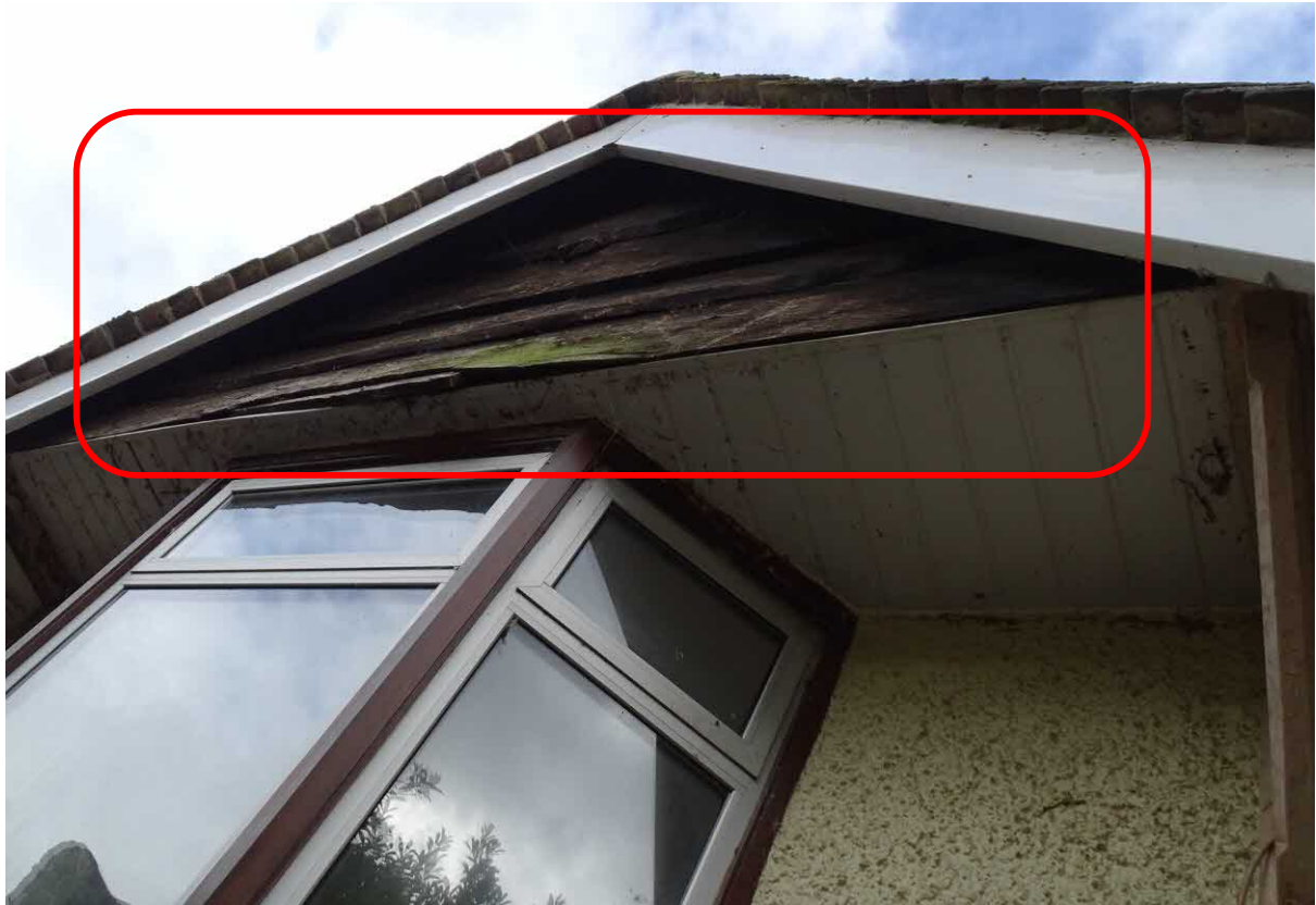
Image 5 – Further gaps of value to bats observed within the vertical timber claddings to the South facing elevation of the property
