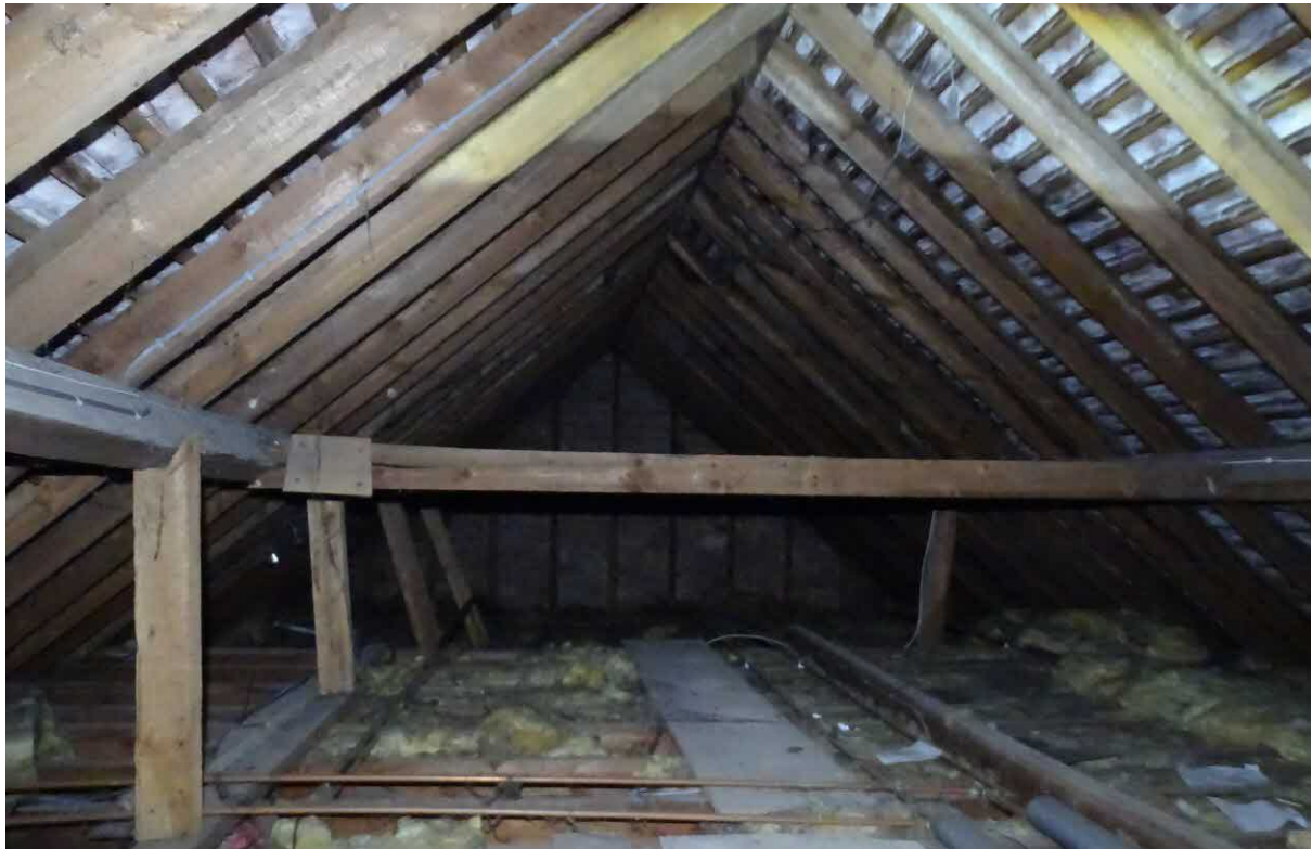
Image 7 – Internal view from within the main roof void spaces of the property
