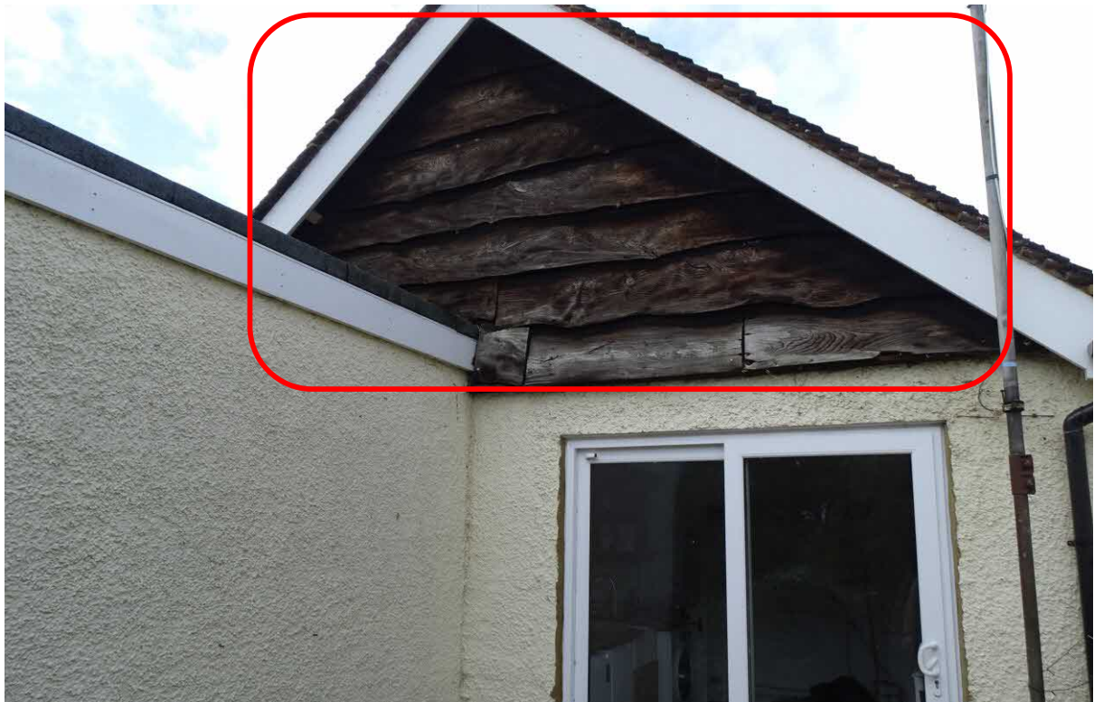
Image 2 – Rear East facing elevation of the property where gaps within the vertical timber cladding look to provide adequate shelter/access opportunities for bats
