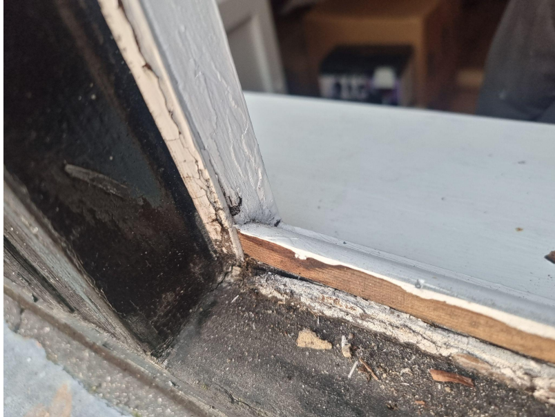
The external mastic is failing and coming away from the window which is allowing the water to enter the casement.
