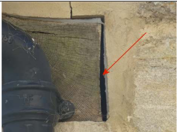
Photograph 6. Gap between the lintel and east wall of the breakfast room
