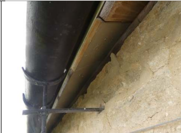
Photograph 14. Thesealed area under the eaves of the garden store
