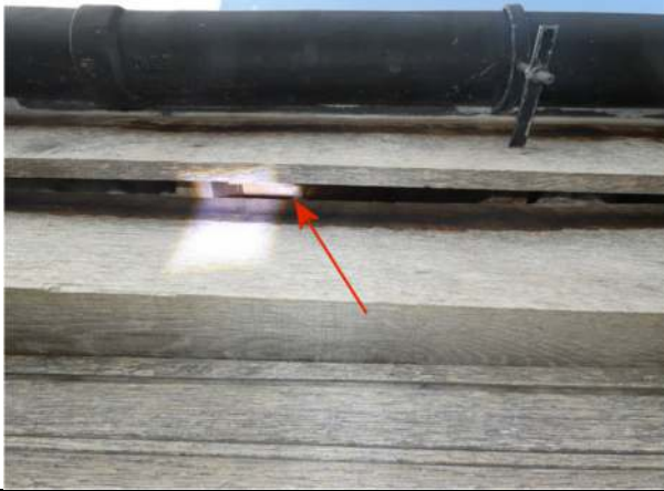
Photograph 7. Opening under the fascia on the south side of the breakfast room
