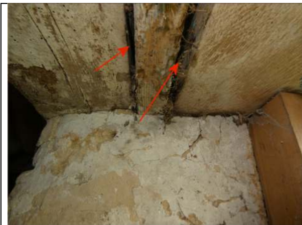
Photograph 17. Crvices in the door lintel of the garden store
