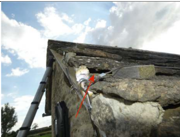
Photograph 11. Example of an opening under a slate in the roof of the garden store
