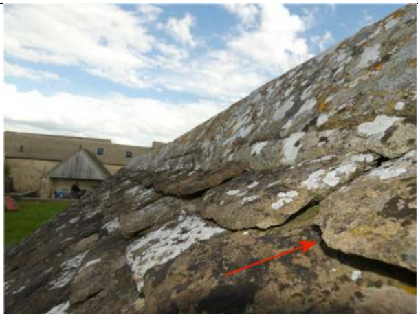
Photograph 12. Further example of an opening under a slate in the roof of the garden store
