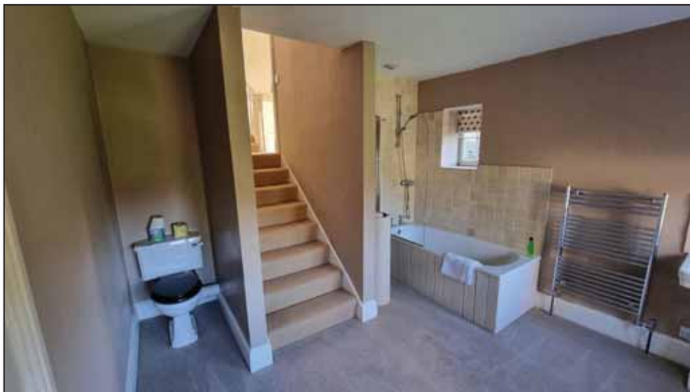
Image 19: Main bathroom showing current access issue
