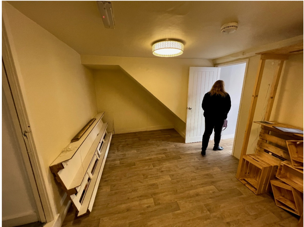
Prior to the work taking place photo showing the position of the range fireplace, stud partition, historic window and trap door to cellar.
