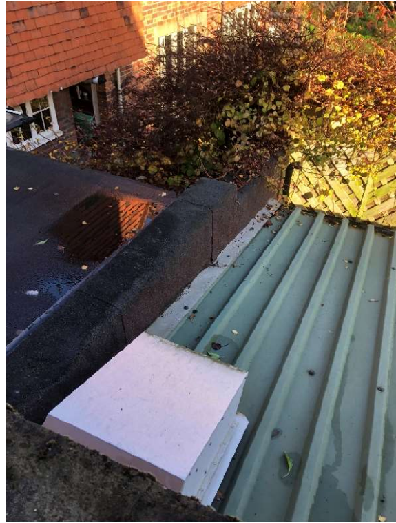
Figure 2: Metal roof of car port and kitchen vent with parapet wall and defective flat roof beyond
