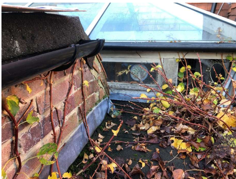
Figure 6: Junction of utility roof with roof over store showing lantern light of No.3 Horsell Grange in background
