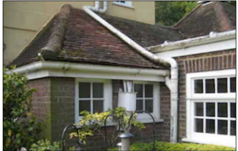
Figure 16: This photograph shows the uncomfortable nature in which the lean-to (G2) roof spans the roof of G1 to reach the northern pavilion roof. The way in which the entire roofs link is suggestive of a secondary, or evolutionary change.
