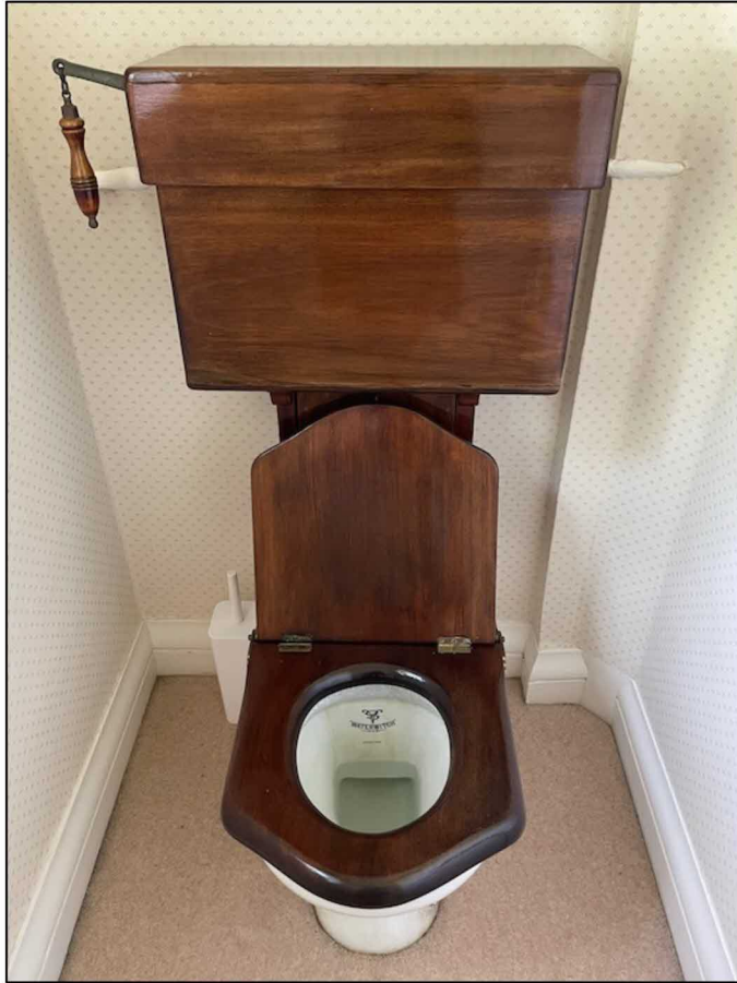
Figure 30: The Waterwitch WC in room F1c. Photographs ©Hubbard Conservation.
