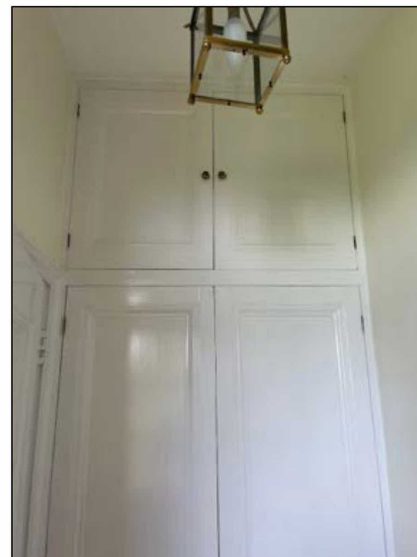
Figure 8: Cupboards and partition to the northeast corner of G3 adjacent to G2.
