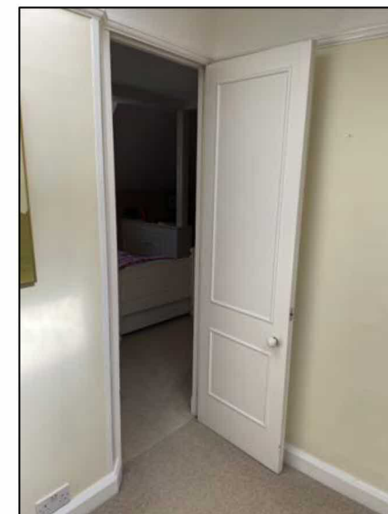
Figure 18: F5 door into F2. Top – east cupboards in S4. Below – door between S4 and S2.
