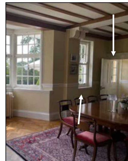
Figure 11: Top – external view of the east elevation. Below – internal view of the door and adjacent window.
