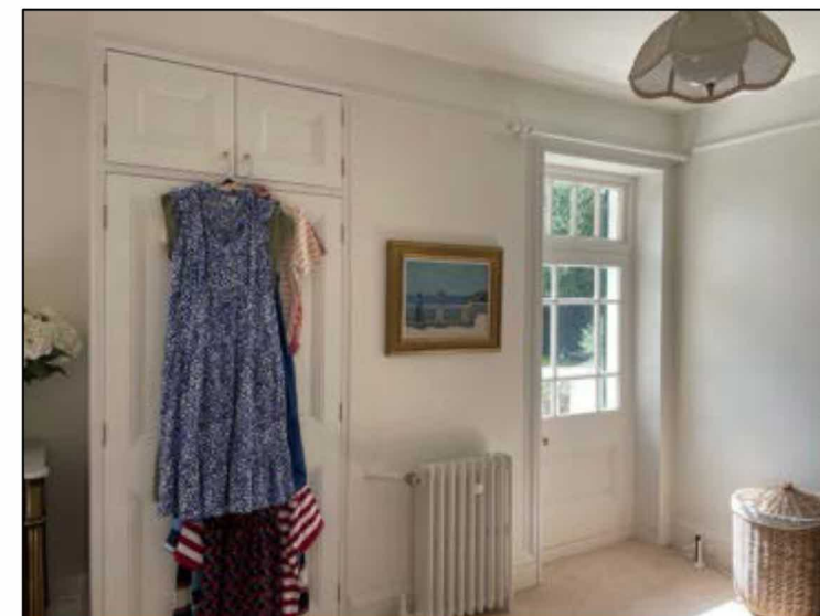
Figure 15: Room F6. Modern cupboard against south elevation blocking window.
