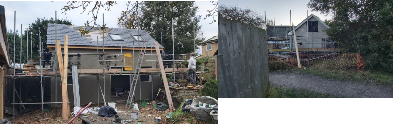
1949.16A Side elevation of current outbuilding under construction (Dec 2023) And inset, 16B rear (footpath) elevation of outbuilding.
