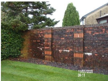
Existing deteriorating boundary wall
