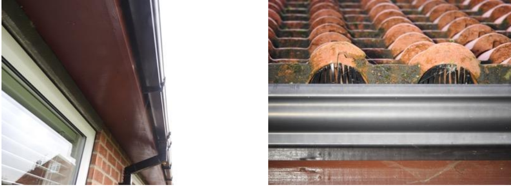
Figs. 14 & 15 Tightly fitting boxed soffits (L) and eaves filler combs (R)
