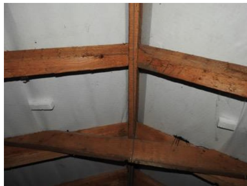
Fig. 16 Cobwebbed ridge of the main roof void
