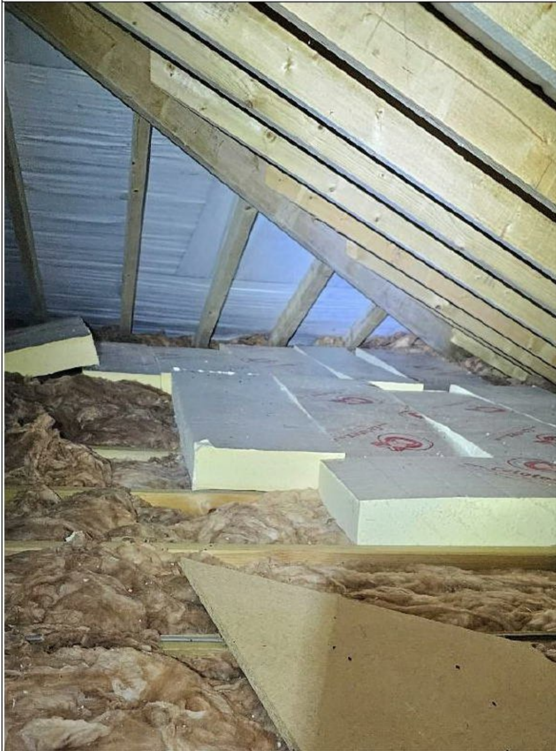
Photograph 23: Loft space tightly constructed.
