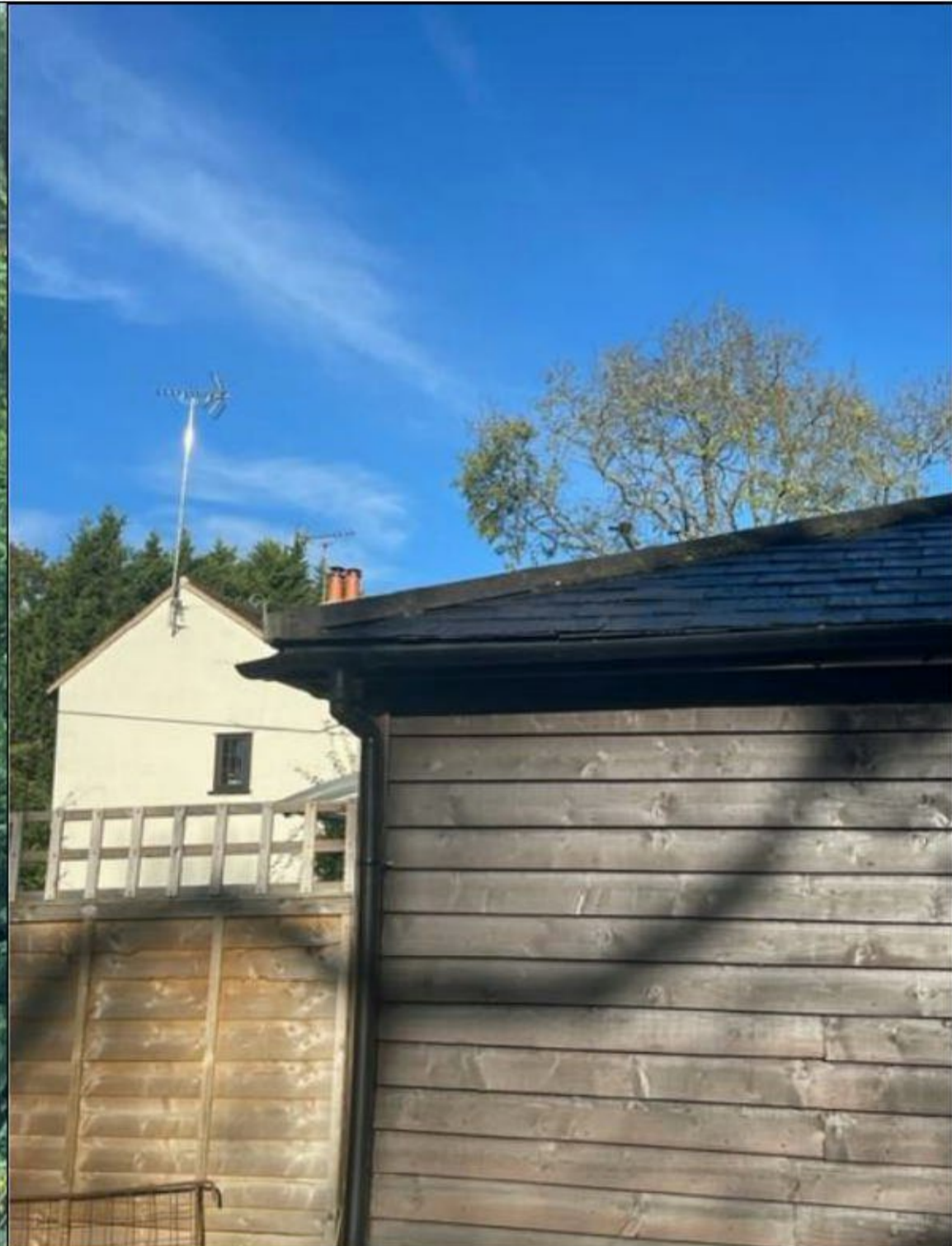
Photograph 14: No gaps around cladding.
