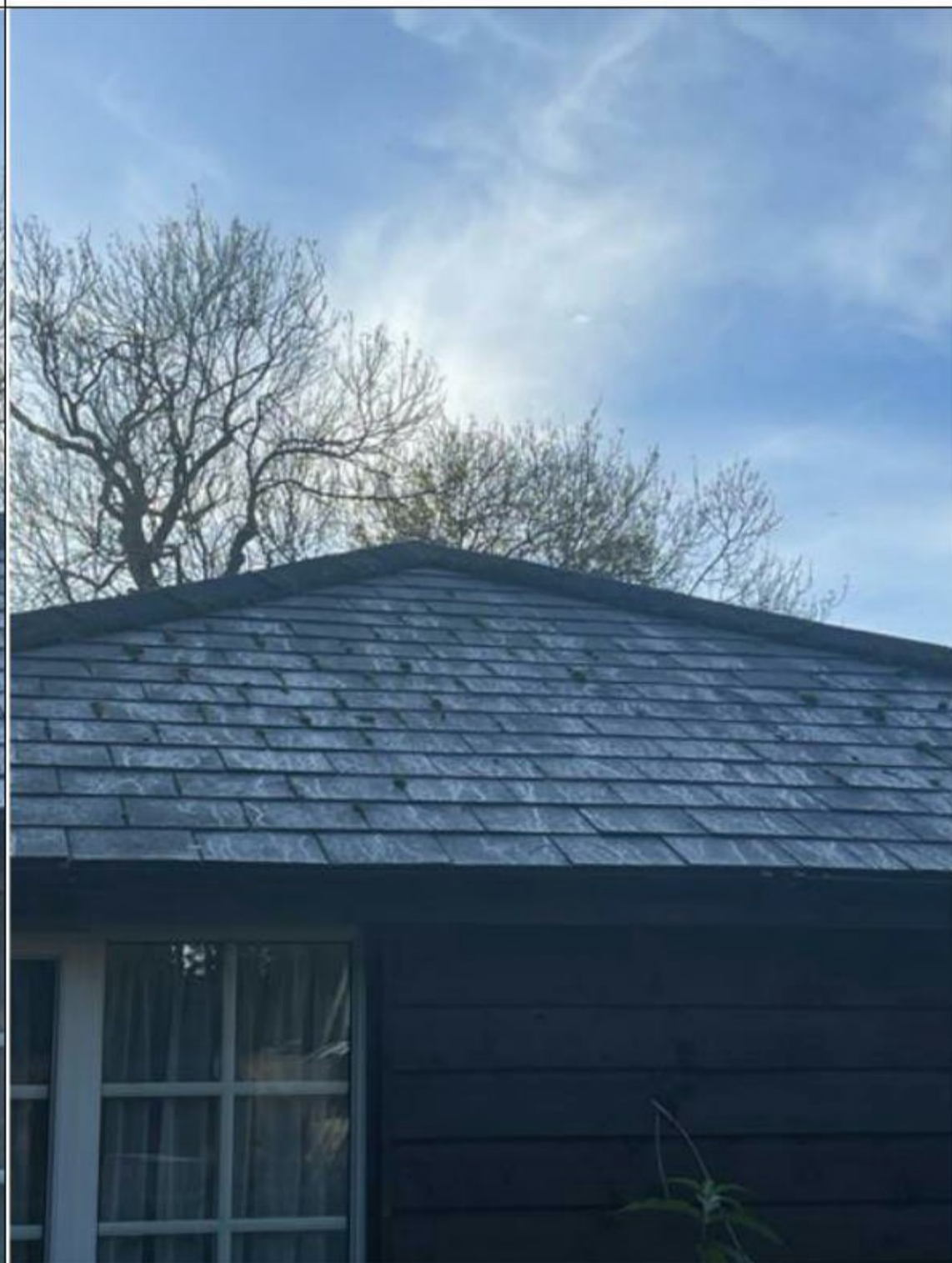
Photograph 20: No gaps under ridge tiles.
