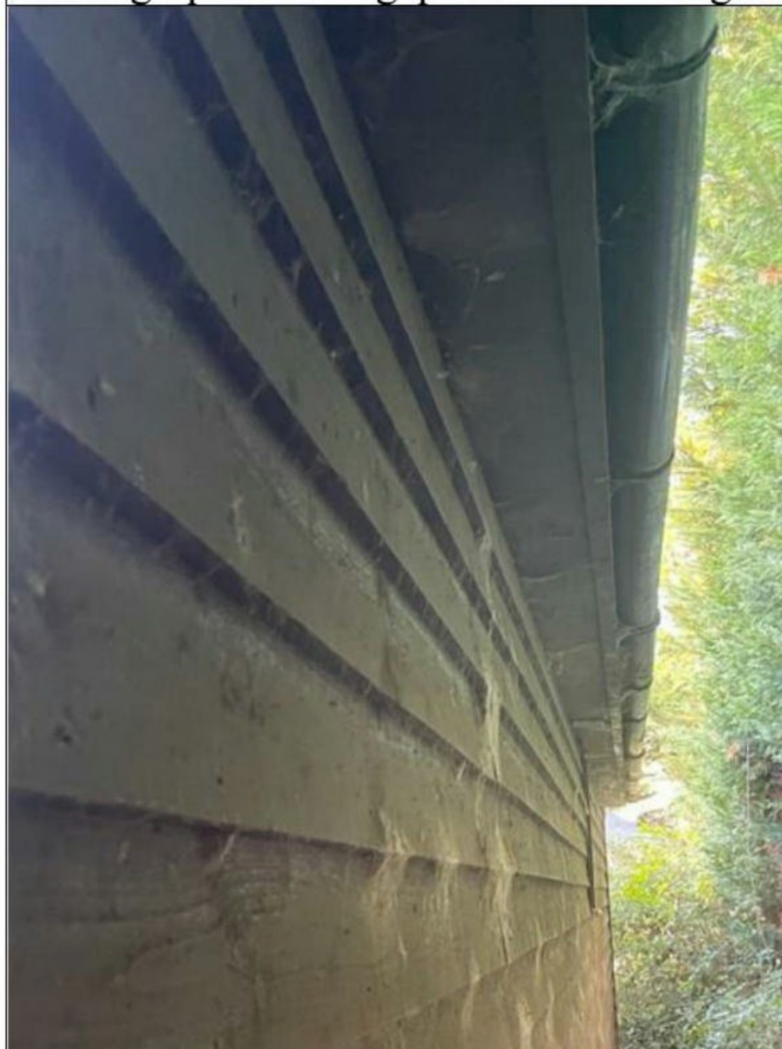
Photograph 15: No gaps around soffits.
