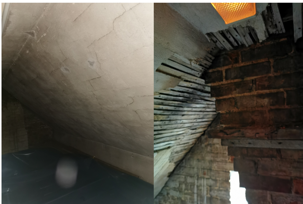
Photos of internal ceilings showing poor general condition.
