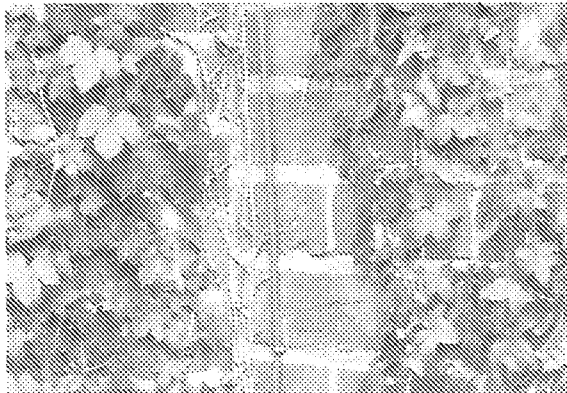
Straight joints in the brickwork are visible which show the house was extended twice along the road side in the 19 th century.
