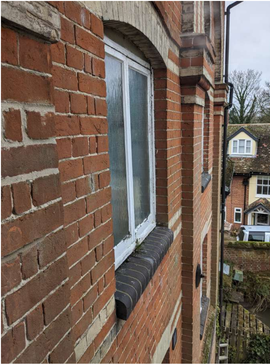
View looking out from Second Floor Landing of Stairwell Block depicting the condition of existing windows
