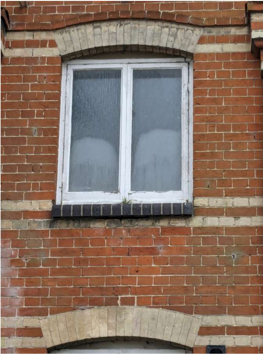
Actual window serving Flat 6, taken from Ground Floor Rear Elevation of Hawks Mill
