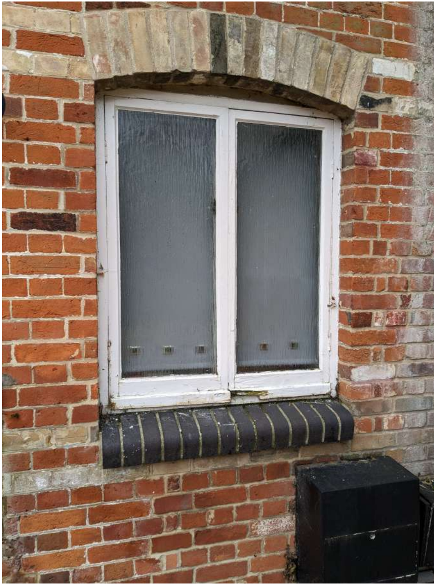
Example of window type, taken from Ground Floor Rear Elevation of Hawks Mill
