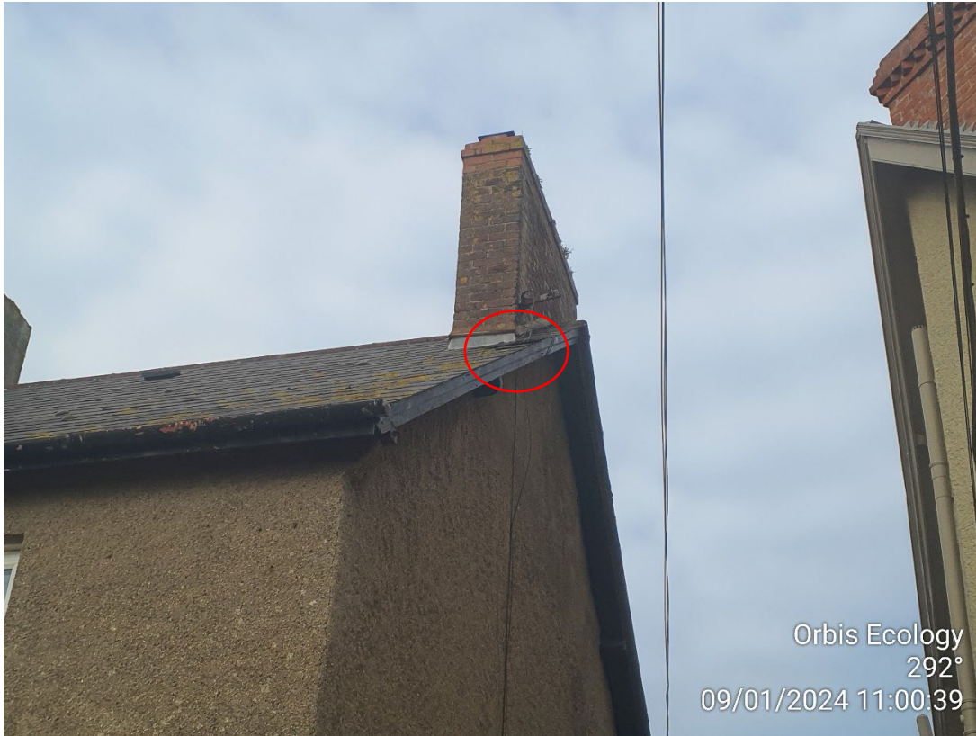
Gap under slate below the chimney on the south elevation
