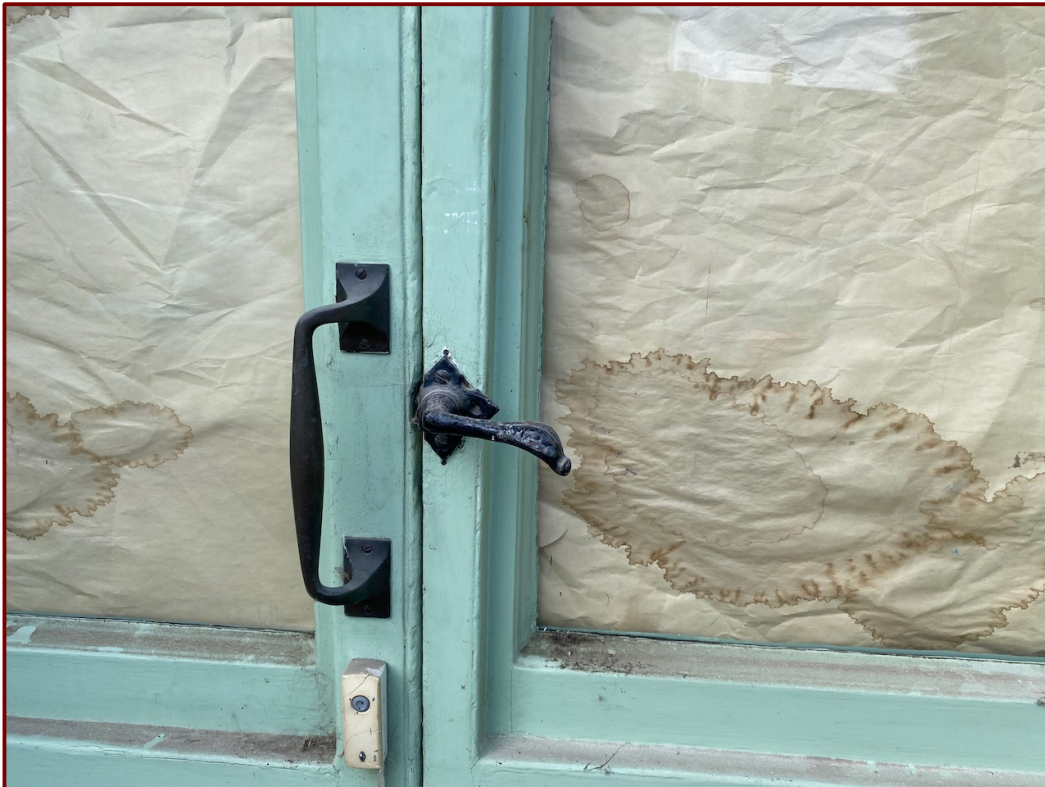
Mismatched and poorly adapted ironmongery.
