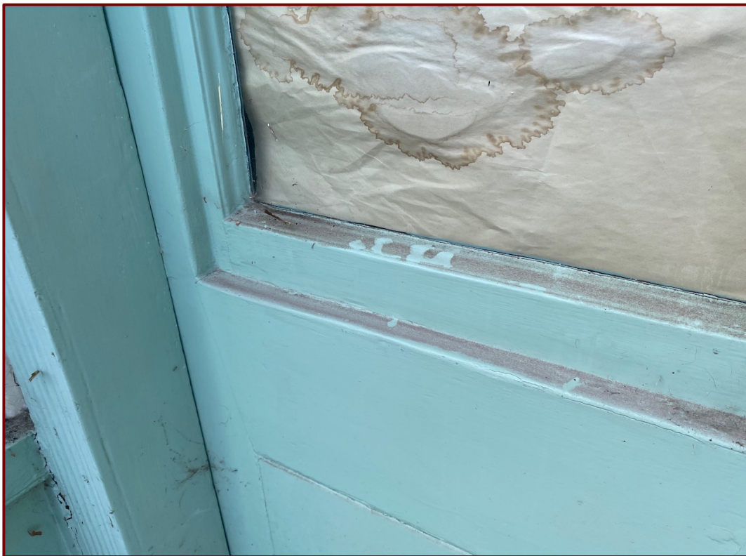
Original gunstock stile doors appear to have has glazed sashes inserted into the original glazing rebate.
