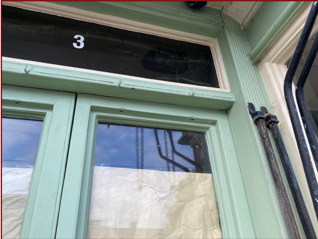
Top of redundant retractable canopy supports.
