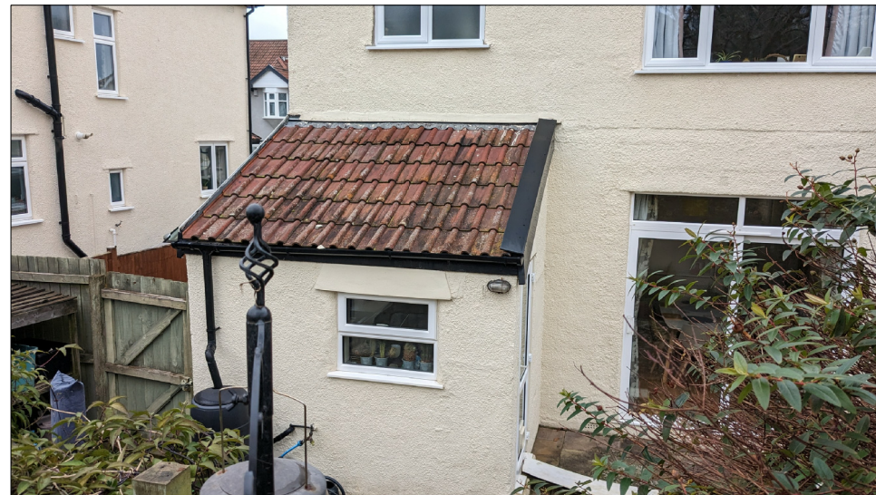
Existing rear projection, to be removed and rebuilt as a full width extension of the same depth.
