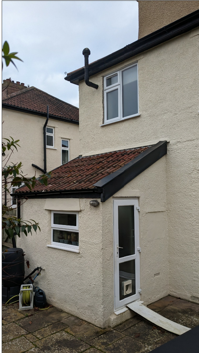
Existing rear projection, to be removed and rebuilt as a full width extension of the same depth. The roof is to be raise slightly as shown on the elevations, to allow better height for the doors at the rear.
