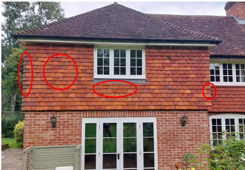
Image No. 02 – B01, western portion of southern aspect. Pipistrelle access points circled in red.
