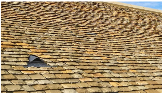
Cotswold Stone effect tiles to pitched roofs
