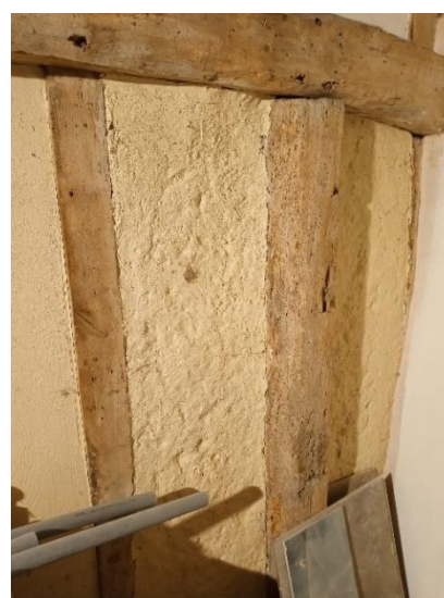
Fig 27. Exposed wattle and daub panel to South end of barn on 1 st floor Plasterboard between rafters
