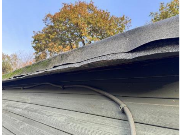
Photo 16: Gaps in Bitumen Felt along Fascia on the South-western Side
