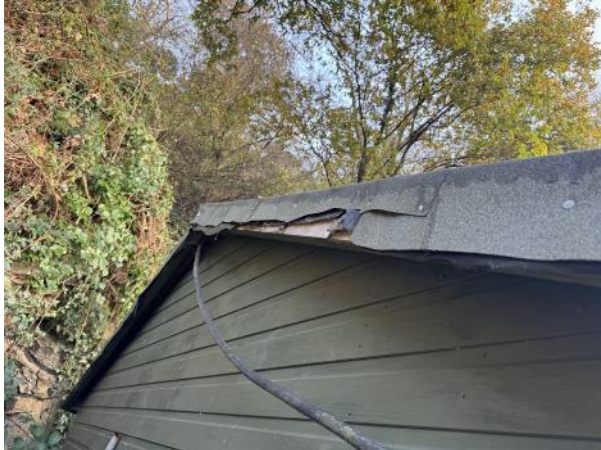
Photo 15: Raised Bitumen Felt on North-western Rear of the Shed
