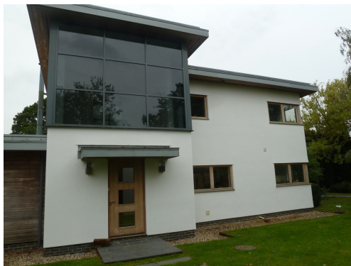
Existing front elevation of main house – painted render, timber cladding and flat roof with metal eaves
