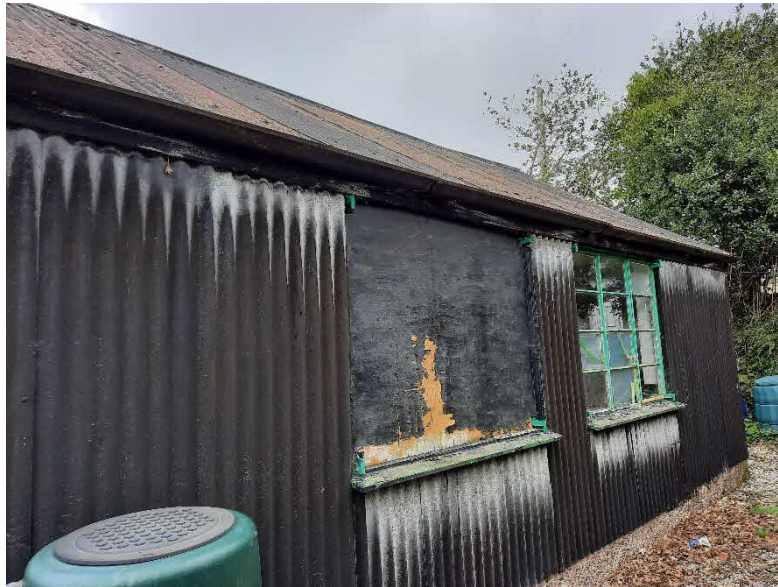
Figure 3: View of the eastern elevation of the garage at Carnon Crescent; one glazed window and one boarded window were present.
