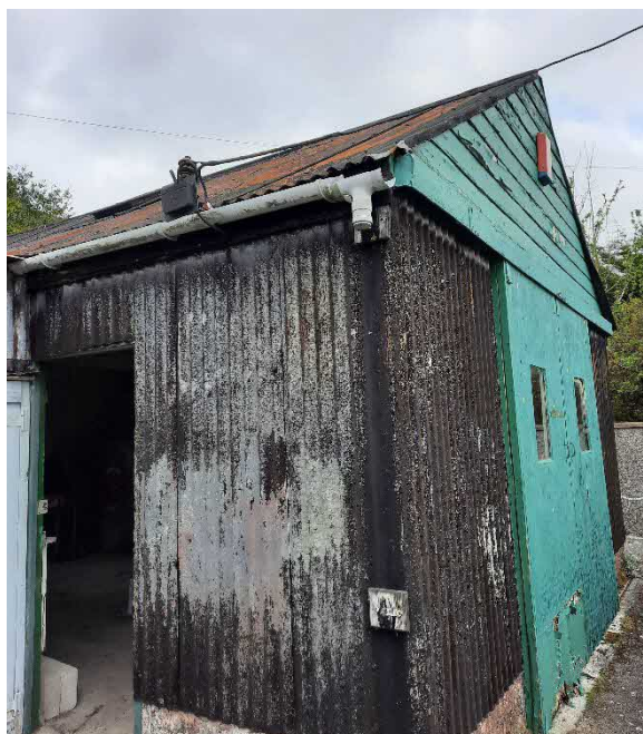
Figure 1: View of the south and west elevations of the garage at Carnon Crescent.
