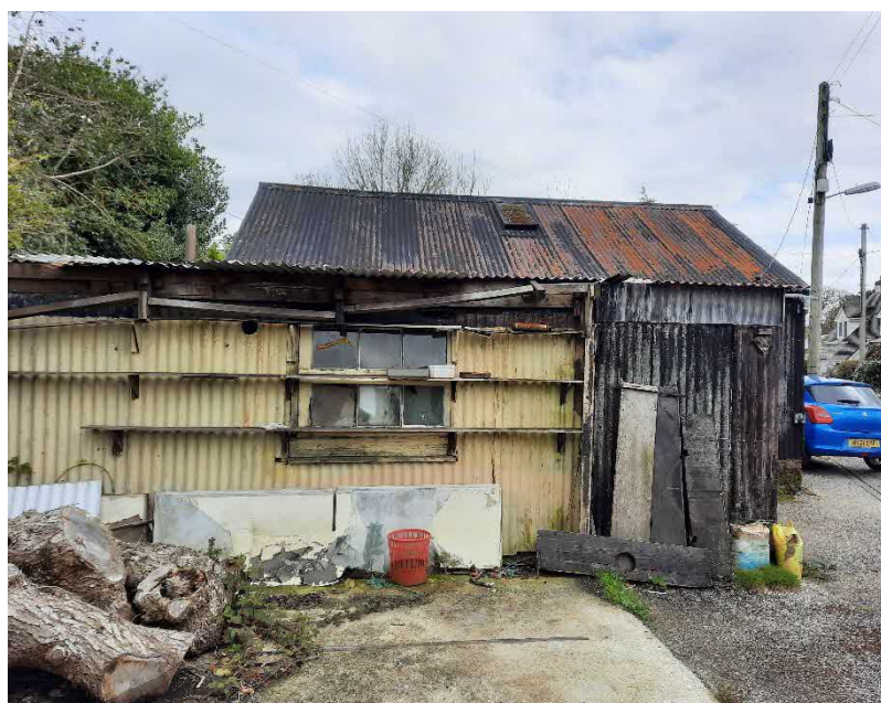
Figure 2: View of the west elevation and lean-to on the garage at Carnon Crescent.
