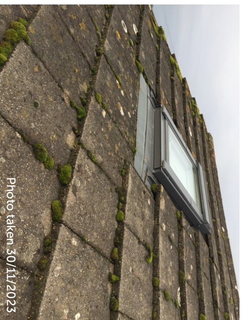
Tight interlocking cement tiles throughout bungalow roof, with existing sky light on southern elevation
