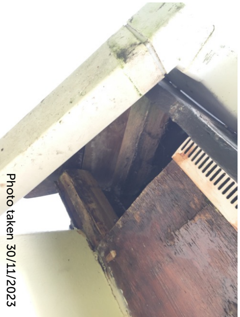
Large cavity in vented soffit at south-western corner of bungalow – affording no roosting potential
