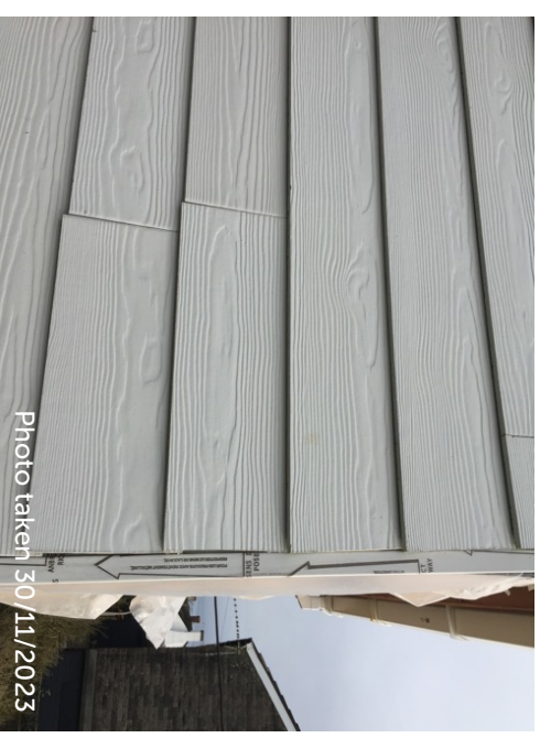
UPVC wood-effect cladding on western elevation of dormer, with plastic sheeting blocking access
