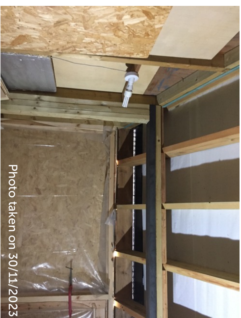
Internal space of dormer, looking south with large window blocked with plywood and plastic sheet
