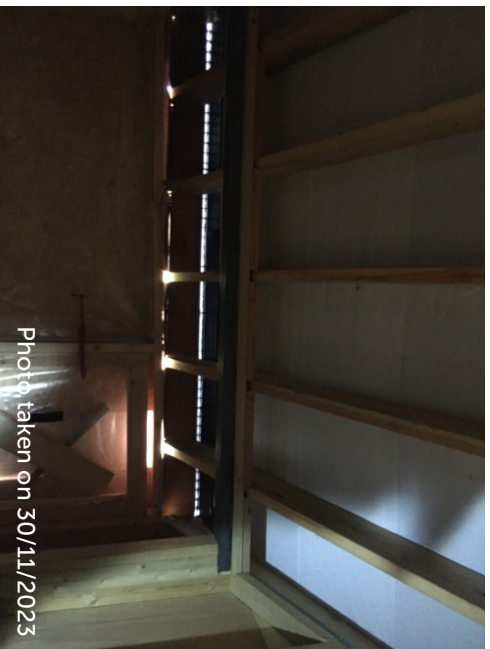
Light ingress at vented grills on southern elevation, affording no potential access for bats
