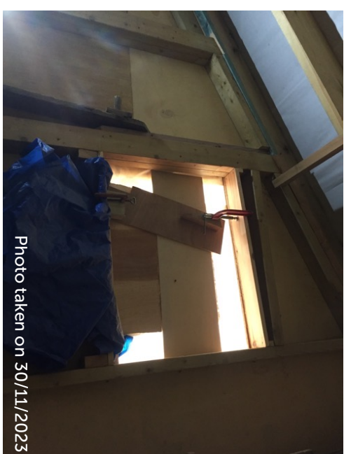
Smaller window opening at western elevation of dormer, blocked with plywood and plastic sheet
