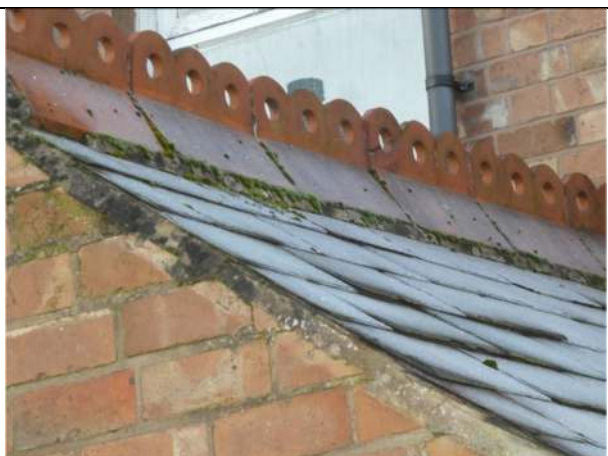
Photograph 6. Example of the slates on the roof of the single-storey rear projection
