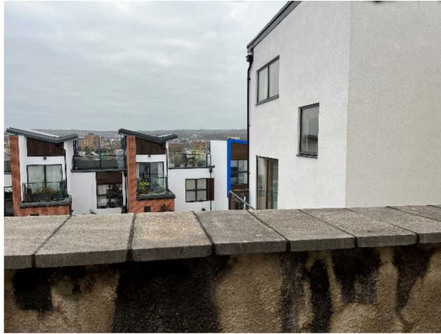
Photo 13. View over the southern boundary wall towards No. 1 Old School Lane and other houses within the development.
