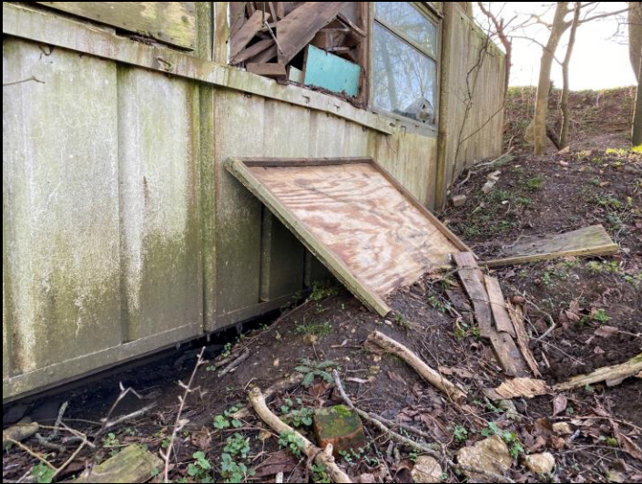
Close up of area near G5, Shipping container/lean-to barn buried
