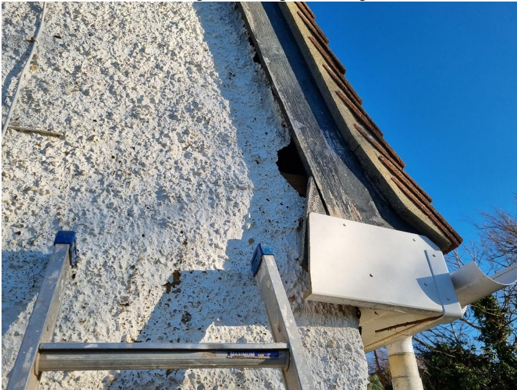
Photo 6 – West gable with large hole near gable end.
