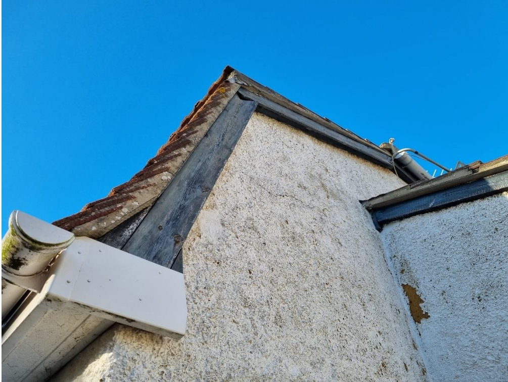
Photo 7 – South-west corner, gaps under barge boards.
