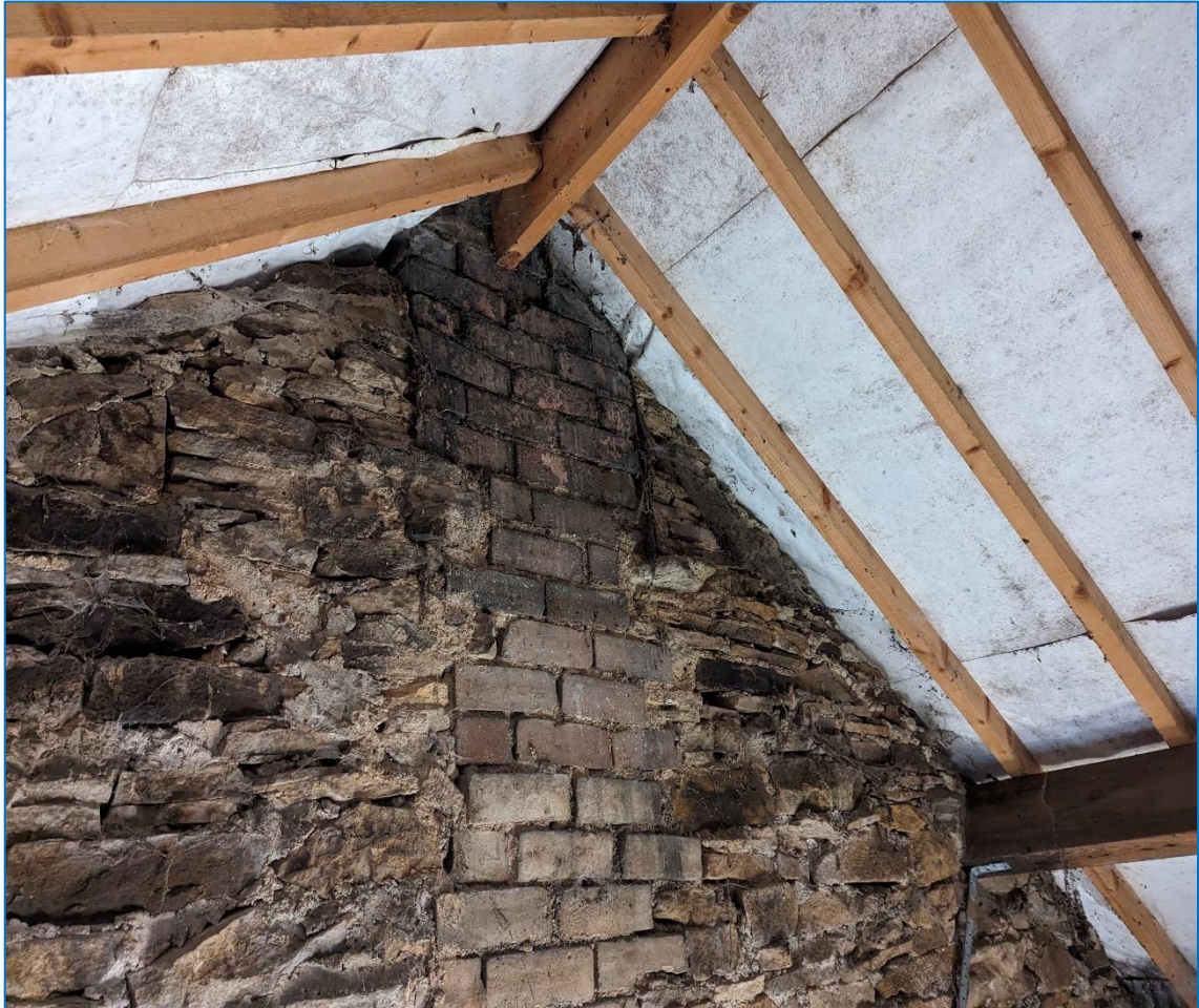
Photograph 12 – Gaps on inside of north gable stone work.
