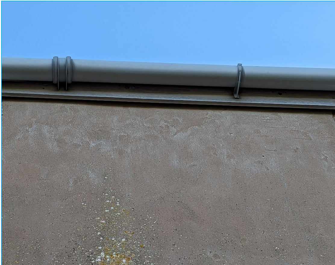
Photograph 9 – Gaps under west elevation fascia boards.
