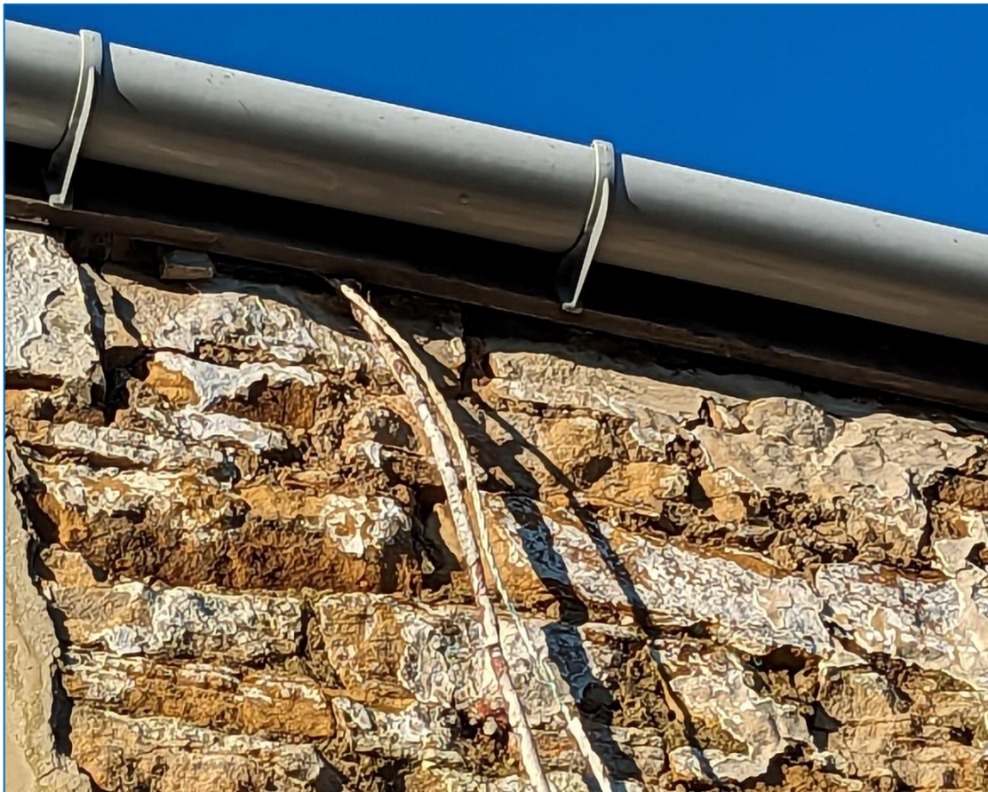
Photograph 7 – More gaps under east elevation fascia boards.
