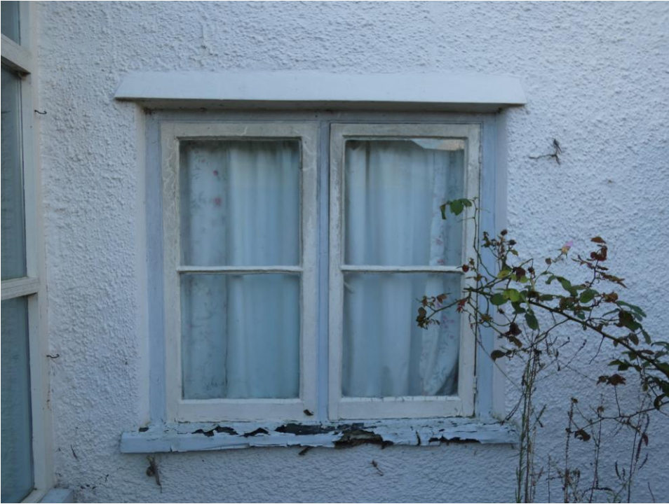
Front GF Righthand side (D) (to be replaced with new as existing)
