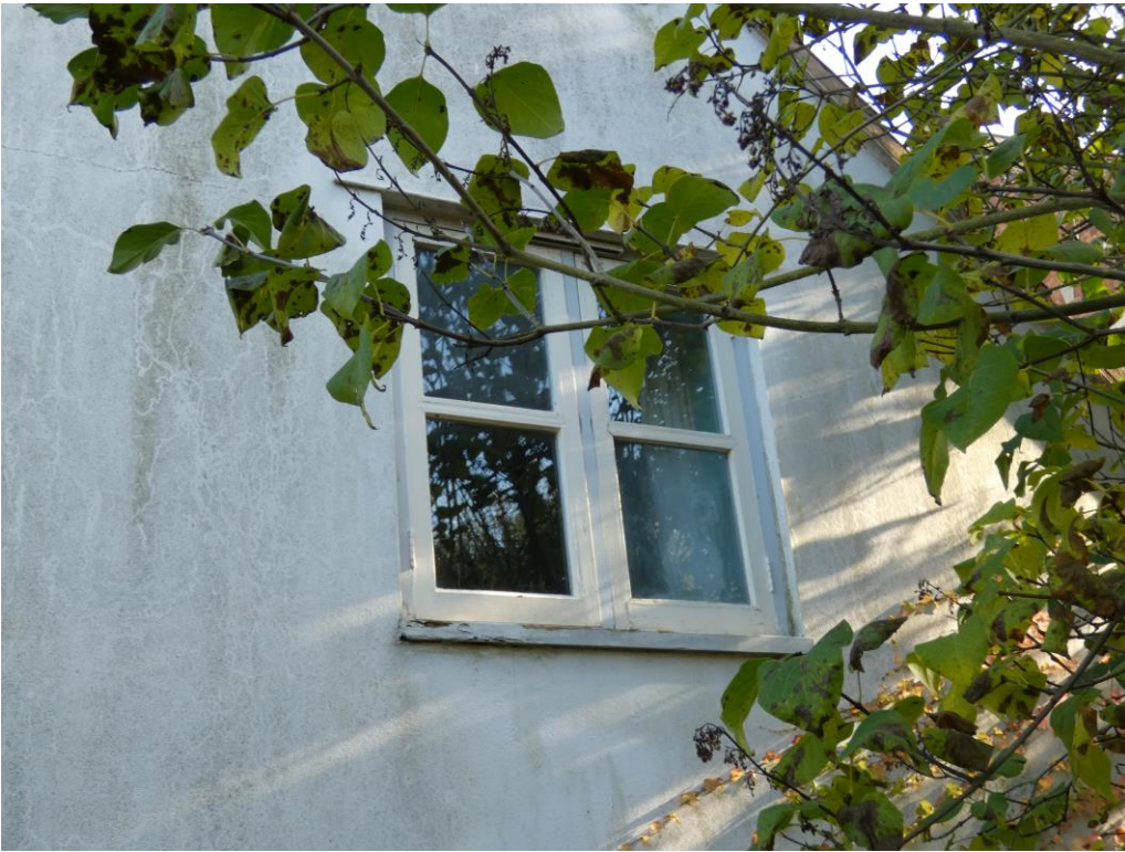
Rear FF Righthand side window (G) (to be replaced with new as existing)
