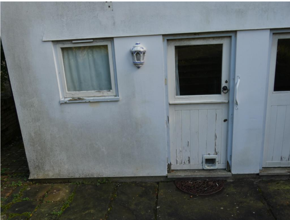
Rear GF Door and window (E) (to be replaced with single window)
