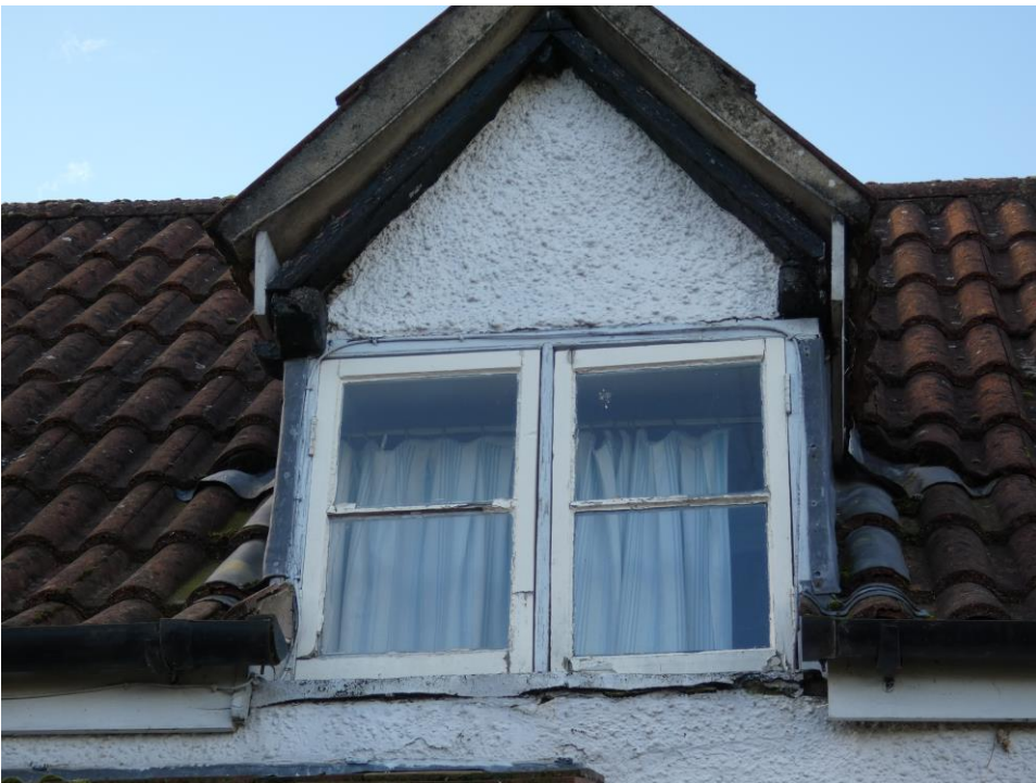
Front FF Righthand Dormer window (C) (to be replaced with new as existing)
