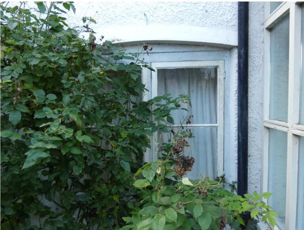
Front GF Lefthand window (A) (to be replaced with new as existing)
