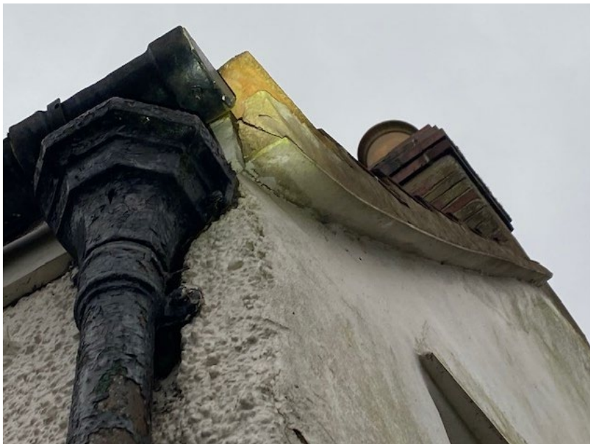
Gap below tiles at wall top of north-east corner of cottage
