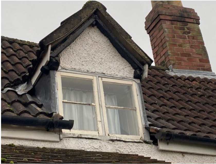
Gaps around dormer window, front elevation
