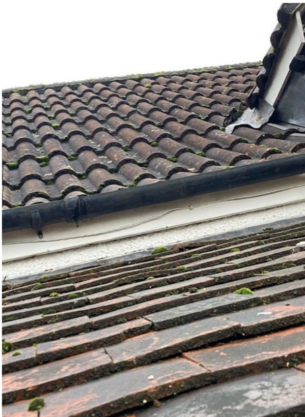
Close view of porch roof gaps
