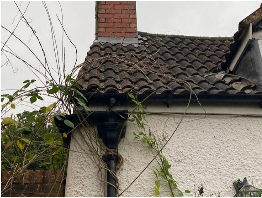
Gaps around dormer and lead flashing on east elevation, south end of cottage
