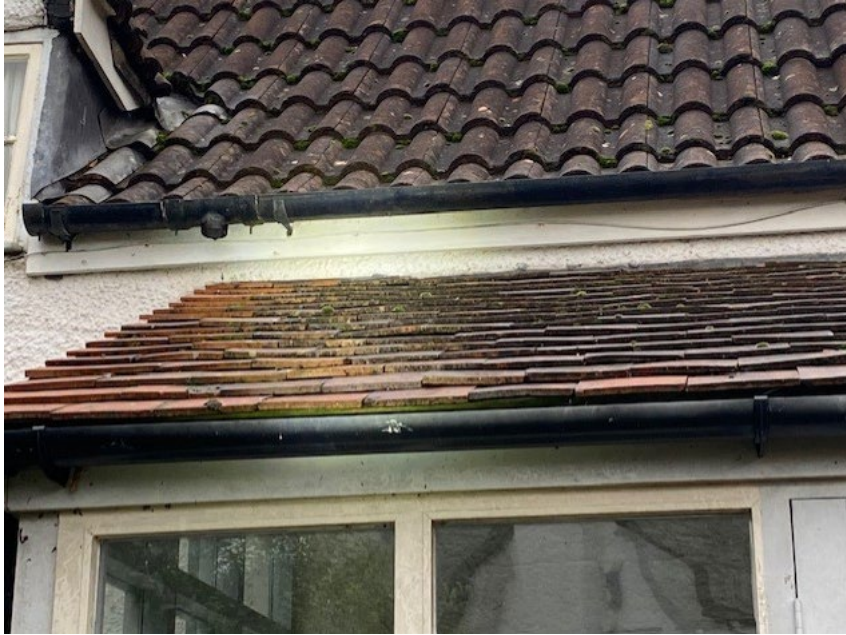
Uneven roof providing small gaps between tiles on porch roof
