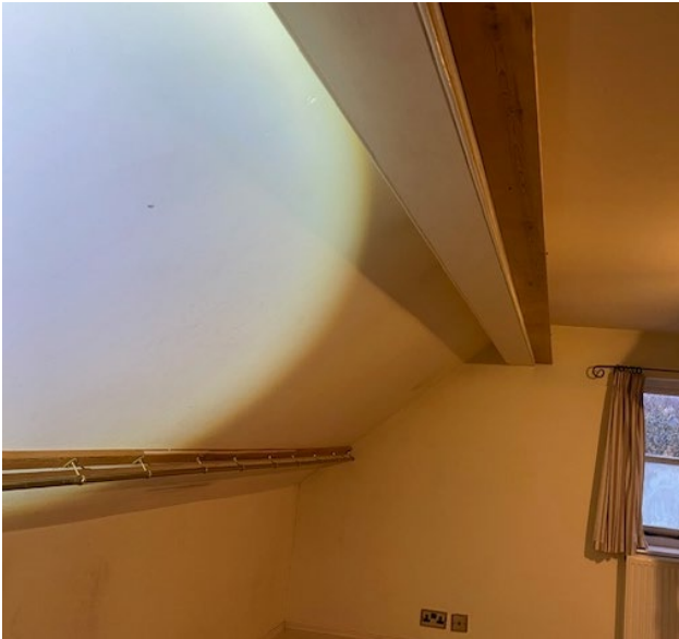
Inside northern rear bedroom illustrating sloping ceiling of part of roof within room
