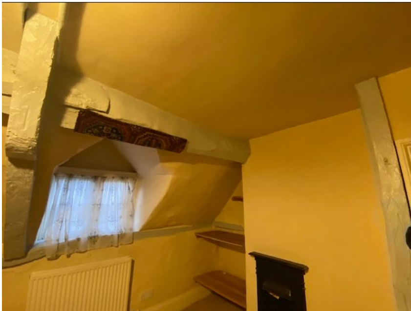
Roof over front of cottage with rooms built mostly into the roof ridge area leaving a small space above with no hatch access
