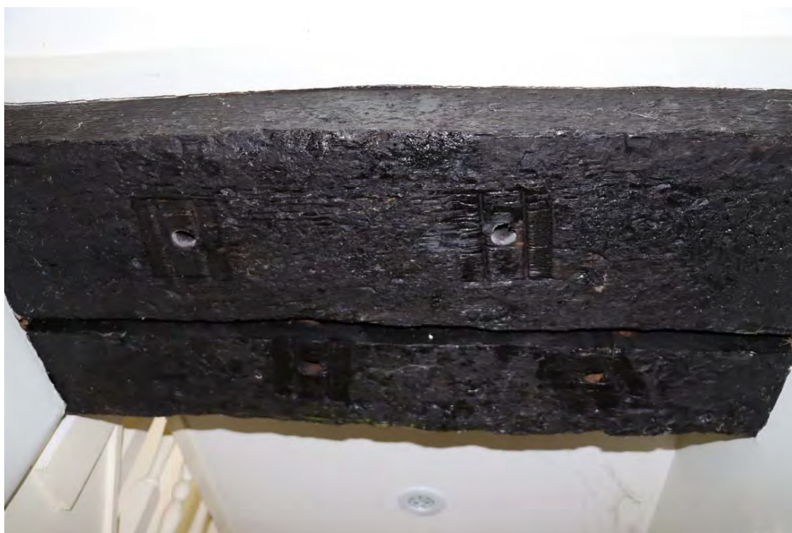
Plate 24: Detail of holes and marks in soffit of lintel over opening between G1 and G4. Similar marks are found on a number of window lintels.
