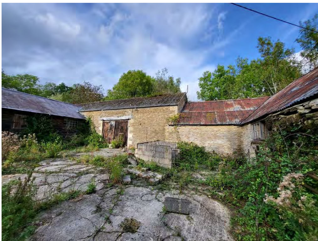
Plate 60: Barn 1 (East), front elevation to courtyard, with Barn 5 to left and Barn 4 to right
