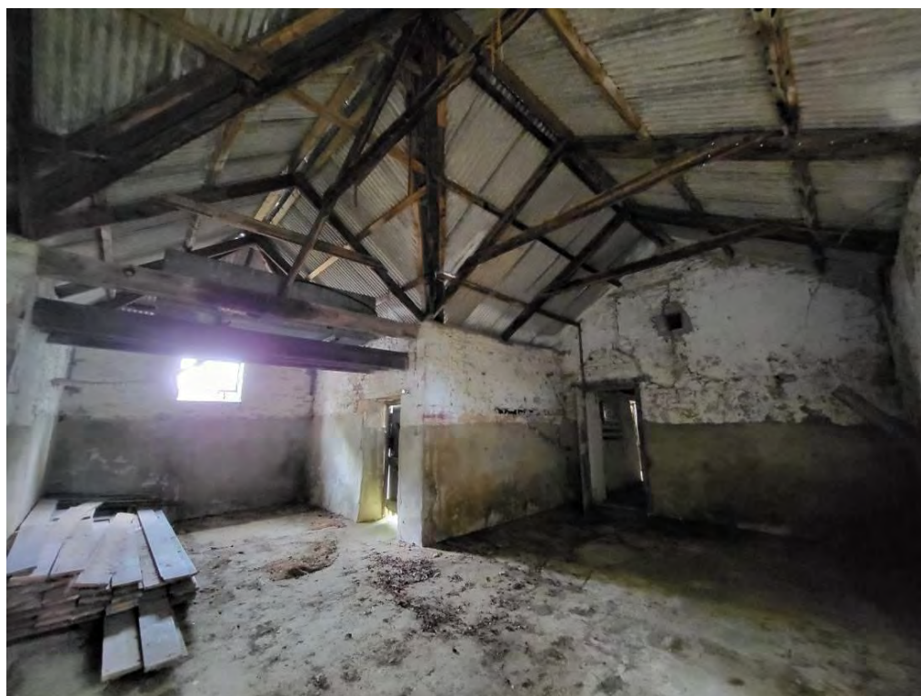
Plate 58: Barn 1 (West), looking south-west towards threshing porch (left) and east wall (right)
