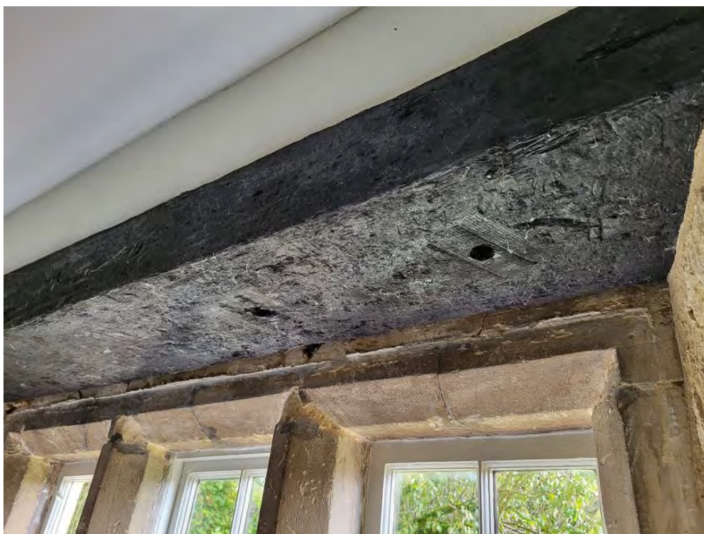
Plate 27: Detail of window lintel with holes and marks, G7
