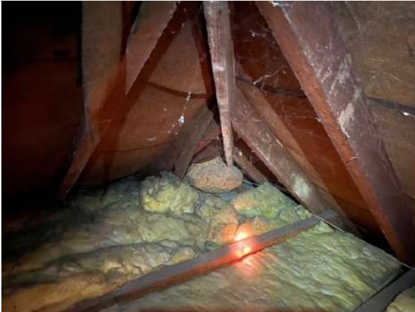
Figure 7. Image showing internal loft space in good state of repair in highest peak of roof. Note in active wasp nest.
