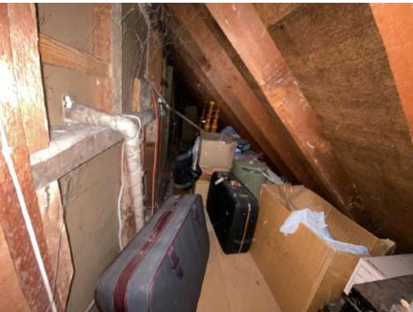
Figure 11. Image showing loft storage space in good state of repair in south-eastern roof space.
