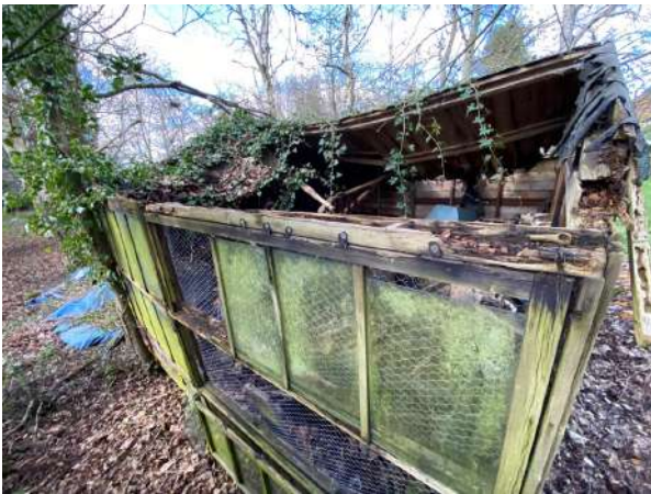
Figure 15. Northern perspective showing garden shed 3. Note defunct roof.
