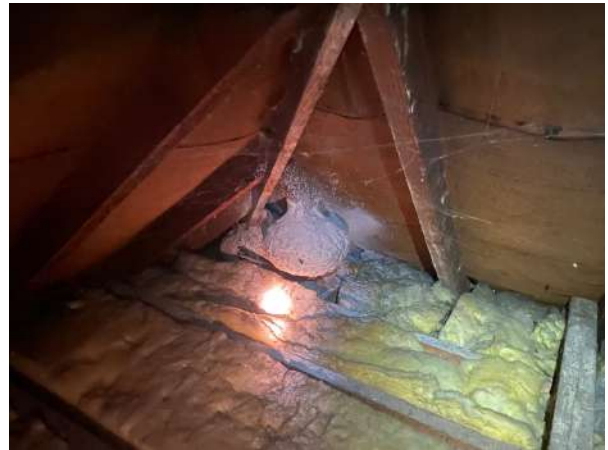
Figure 8. Image showing internal loft space in good state of repair in highest peak of roof. Note in active wasp nest.
