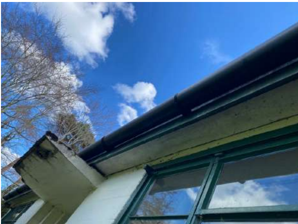
Figure 5. North-westerly perspective showing wooden fascia in good state of repair residential property to be demolished under proposed scope of works.
