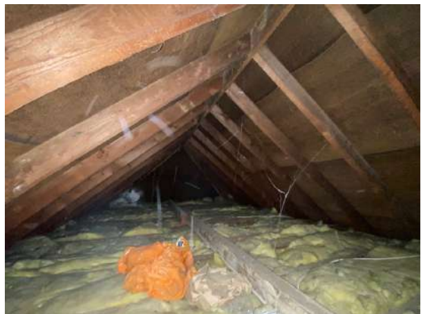
Figure 6. Image showing internal loft space in good state of repair in highest peak of roof.
