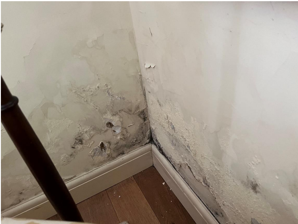
16 – INTERNAL DAMP PENETRATION
