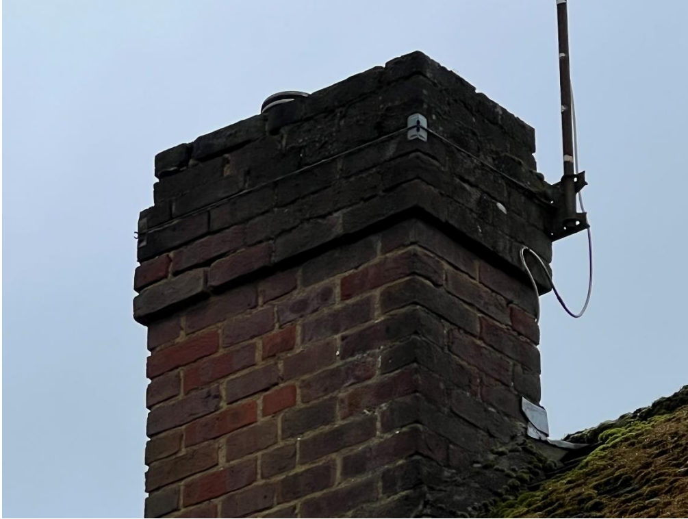
11 – ERODED BRICK JOINTS
