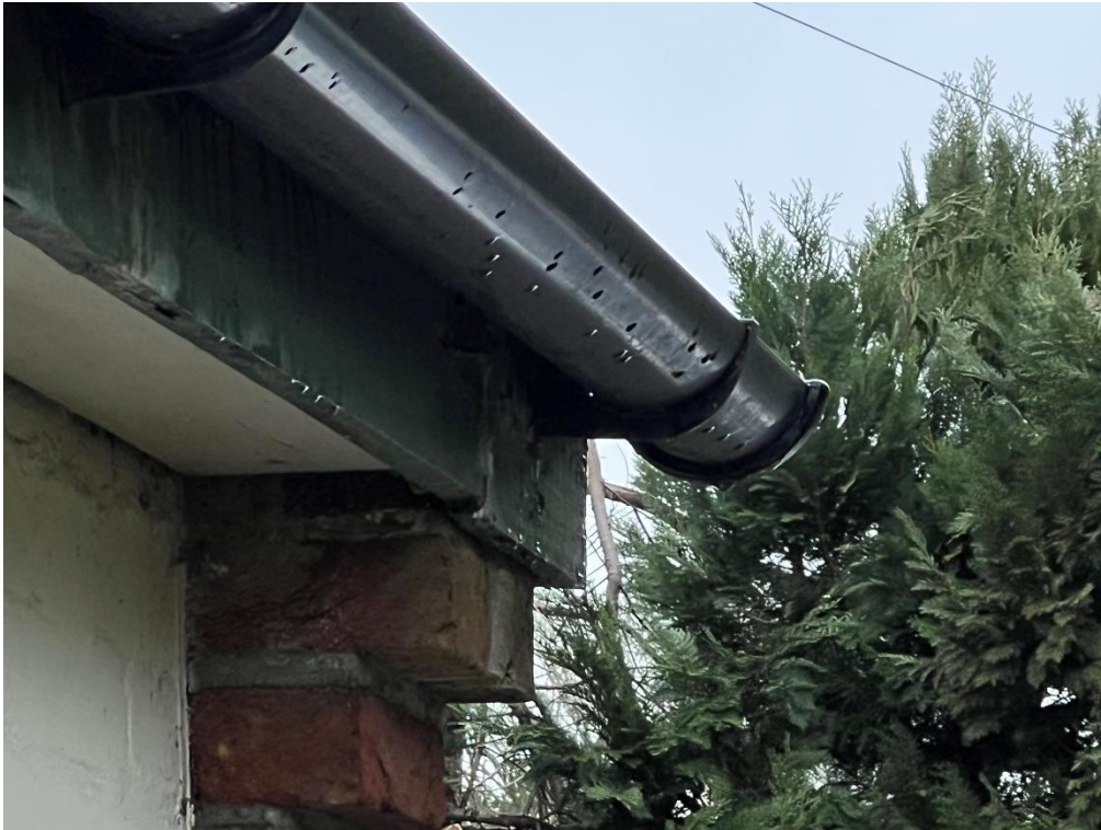
15 – DEFECTIVE RAINWATER GOODS
