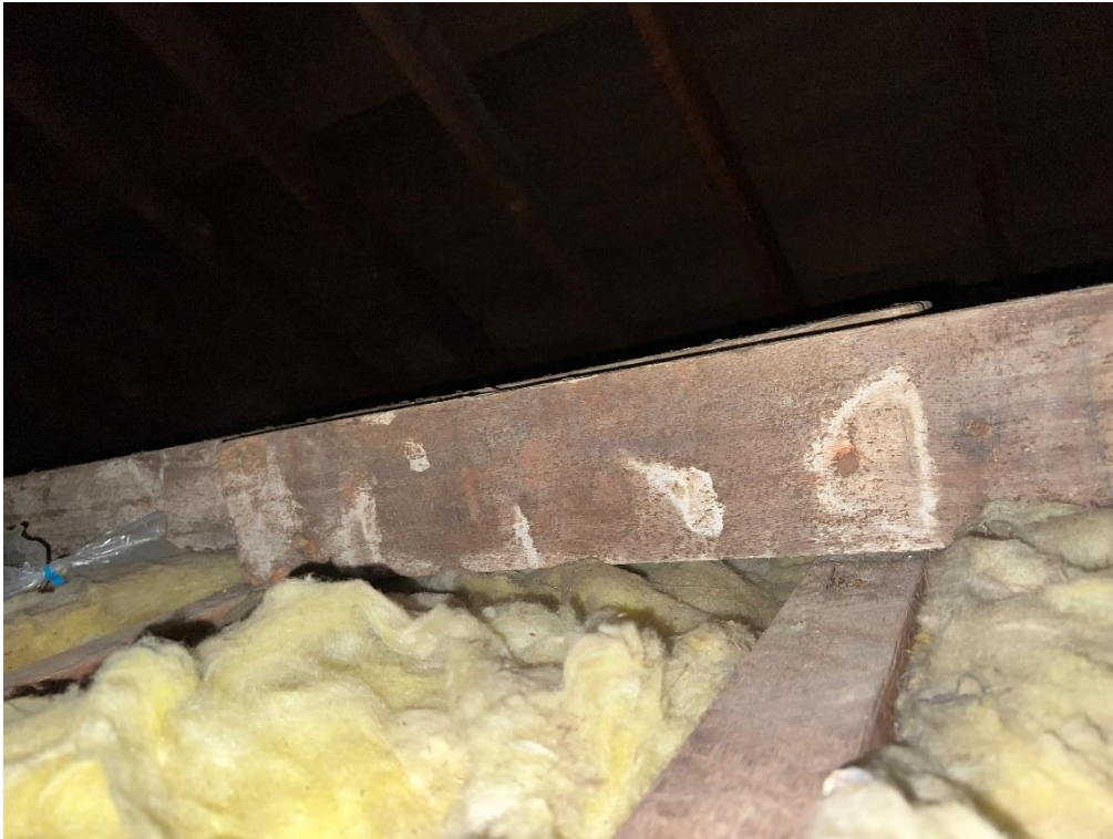
23 – ROOF TIMBERS EARLY SIGNS OF DECAYS
