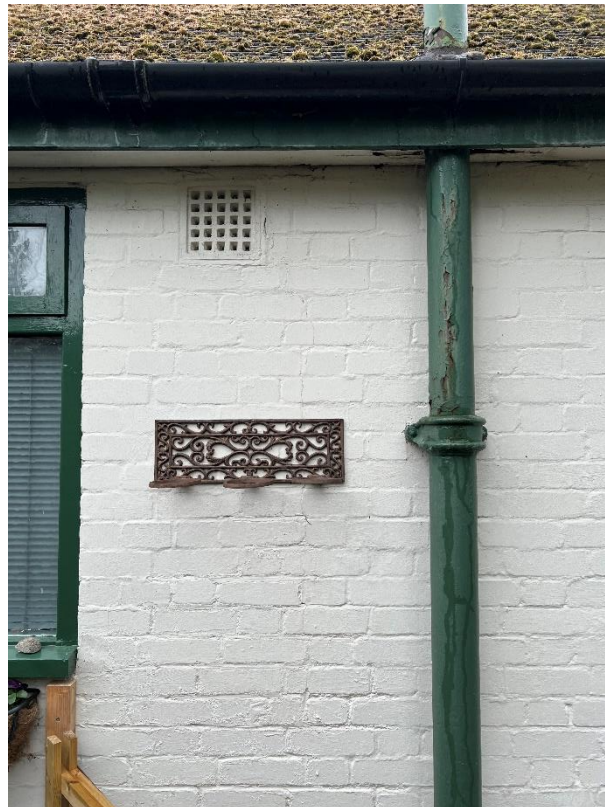
10 – CORRODED SOIL STACKS
