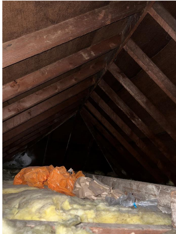
19 – ROOF TIMBERS EARLY SIGNS OF DECAYS
