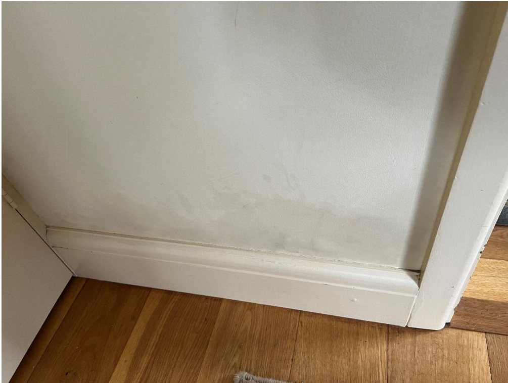
17 – INTERNAL DAMP PENETRATION
