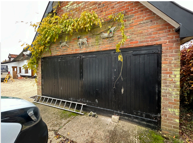
▲ Extract of existing garage doors which are to be replaced.
