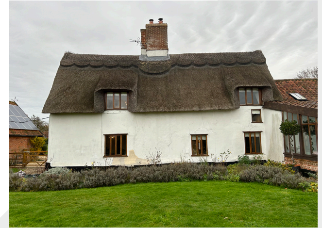
▲ View of rear elevations which is to be affected by the render works.
