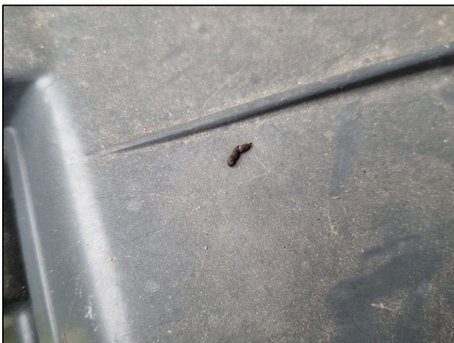
b) Bat dropping found on bin in open bay.
