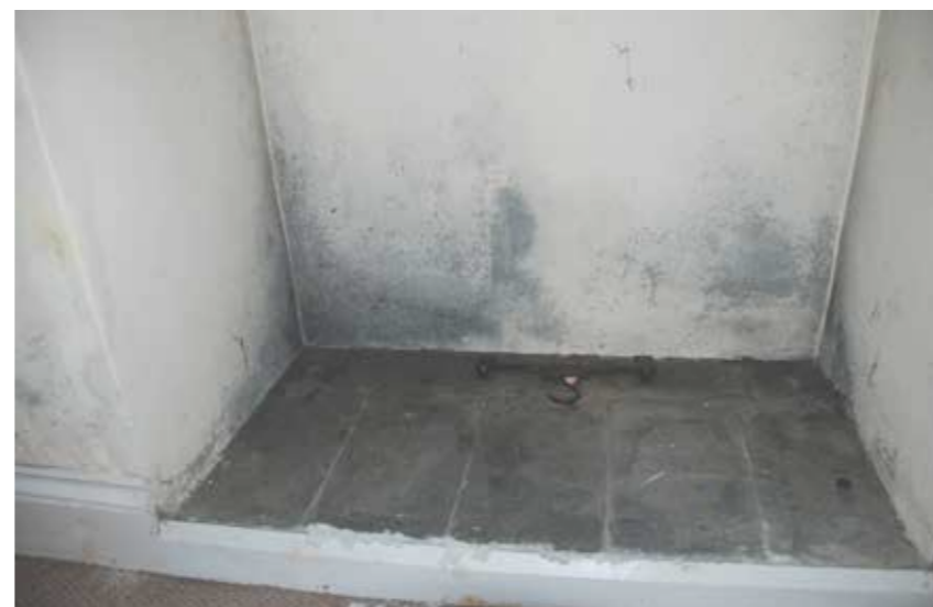
EVIDENCE OF BLACK MOULD AND SALTS WITHIN DINING ROOM FIREPLACE
