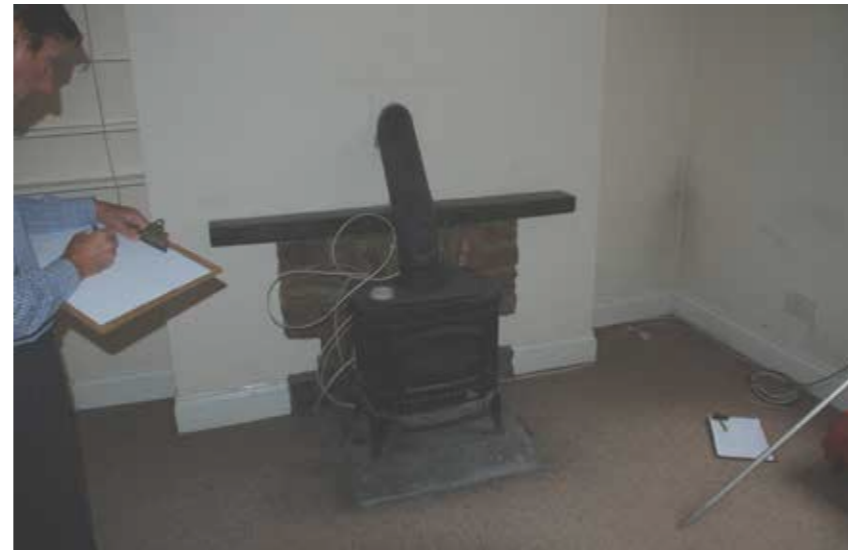
WOOD BURNING STOVE WITHIN LIVING ROOM
