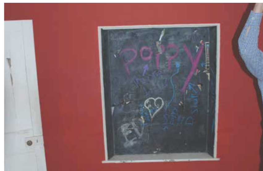
BLOCKED UP WINDOW WITHIN BEDROOM 2
