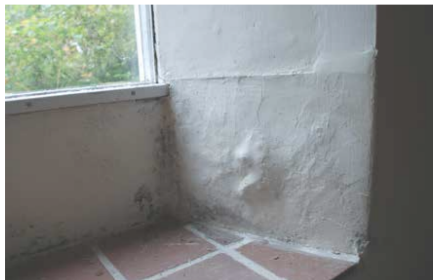
EVIDENCE OF BLOWN PLASTER TO DINING ROOM WINDOW REVEAL
