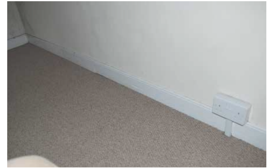
EVIDENCE OF BLOCKED UP WINDOW WITHIN BEDROOM 1
