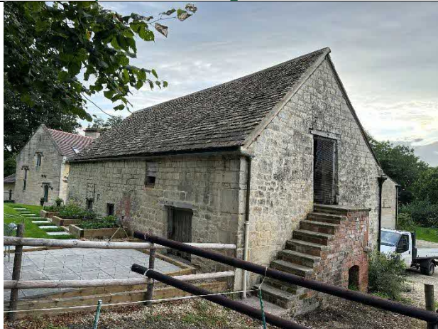
Photograph 3 – South east corner of building. Window with flight access can be seen in centre of image
