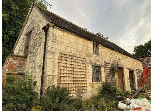
Photograph 2 – North east corner of the building. The concrete tiles that can be seen in this image will be replaced with stone tiles
