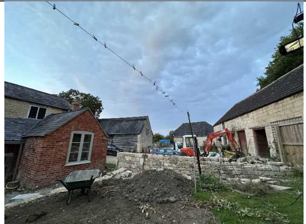
Photograph 4 – Distance between the Cider Barn (right of image) and the main house at Gastrell Farm. The wall that can be seen in the centre of the image has now been completed; however it is only marginally higher than what can be seen already
