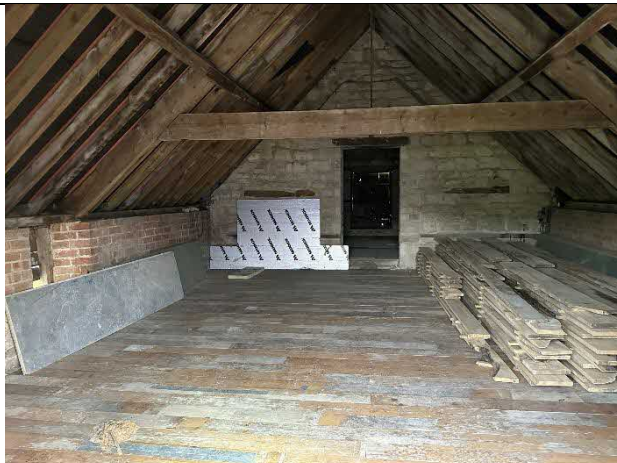
Photograph 5 – Eastern end looking west of first floor/roof space. Window with flight access can be seen to left of image
