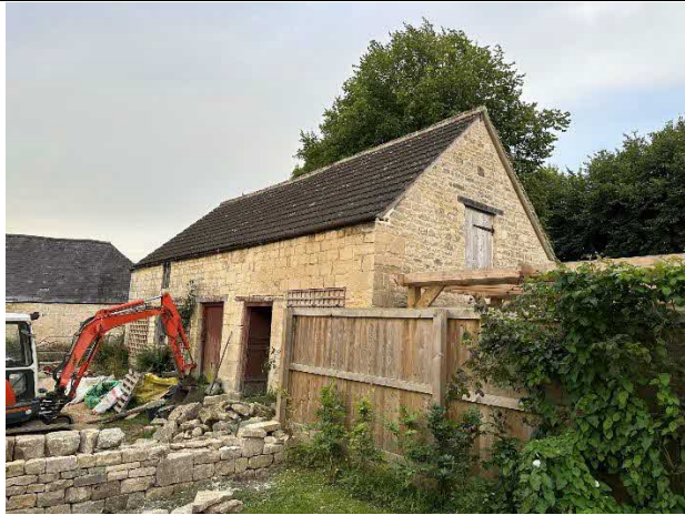
Photograph 1 – North west corner of building. Doorway to the proposed mitigation roosting space within western ground floor can be seen open in this image
