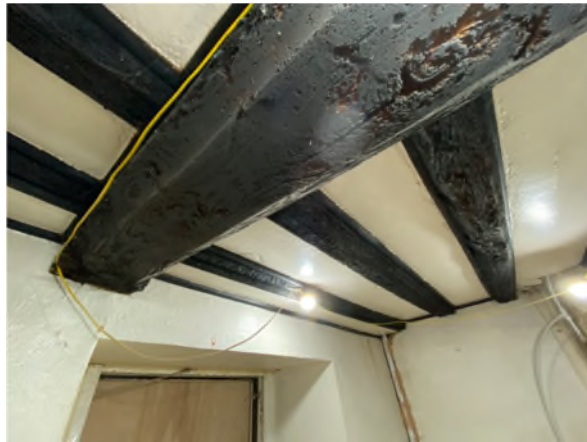
Figure 8: Detail of the axial beam and joists on the ground floor of Phase 1
