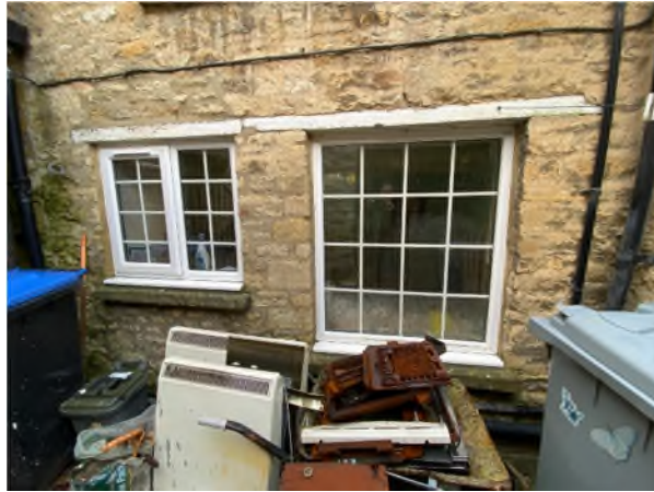
Figure 17: Upvc windows on the ground floor of the south elevation of Phase 2
