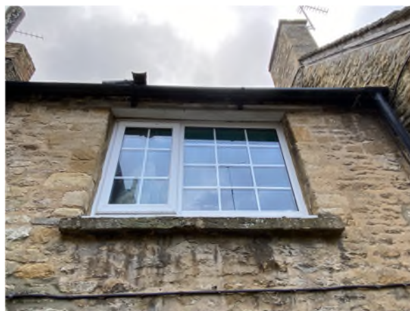
Figure 18: Upvc window on the first floor of the south elevation of Phase 2
