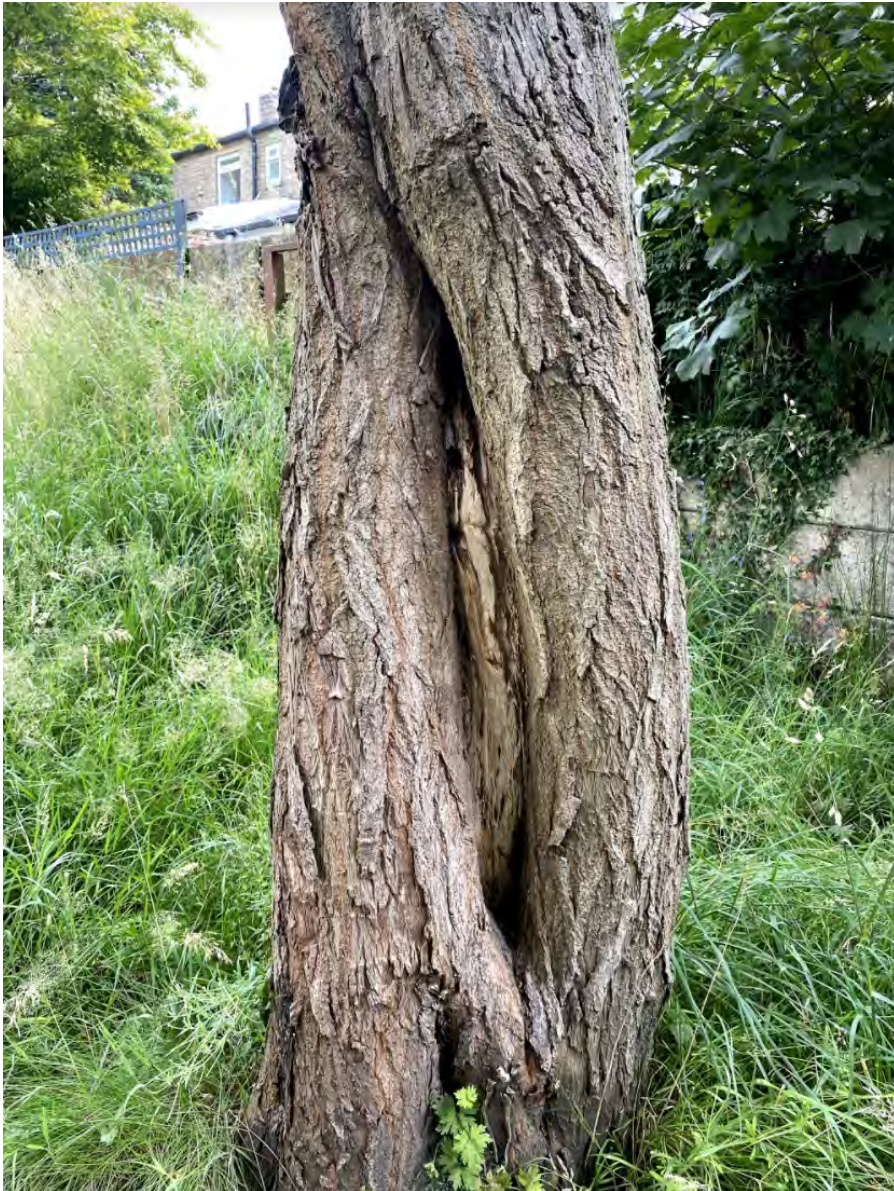
Photographic plate showing a large wound on the stem of tree T3. (ROAVR, 2021)
