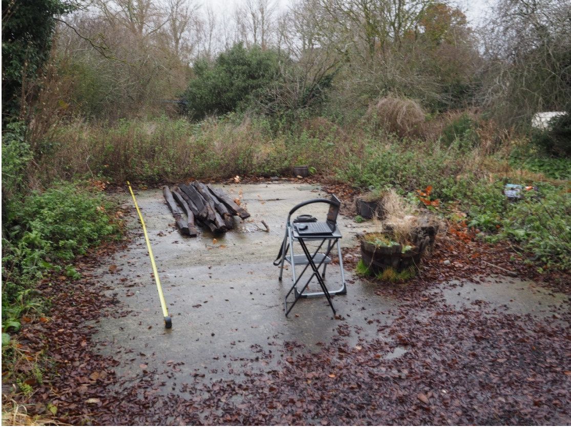
Figure 2: Concrete slab to the rear garden of Meadow Cottage looking South. (Location of previously demolished shed).
