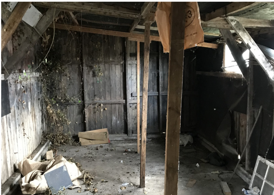
Figure 6: Interior of demolished shed in the curtilage of Meadows Cottage. Note the temporary propping introduced to try and stabilise the structure.
