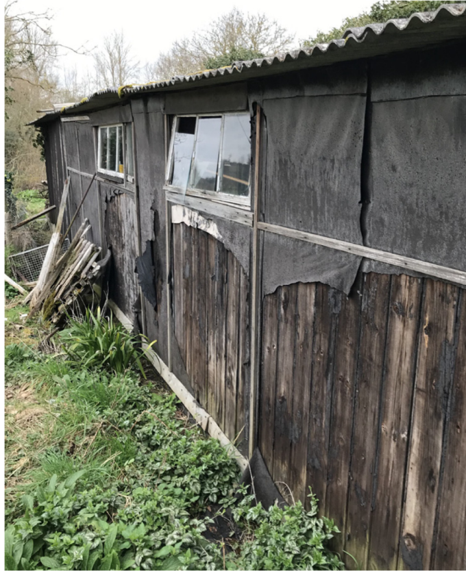
Figure 5: Looking South at previously demolished shed in the curtilage of Meadows Cottage
