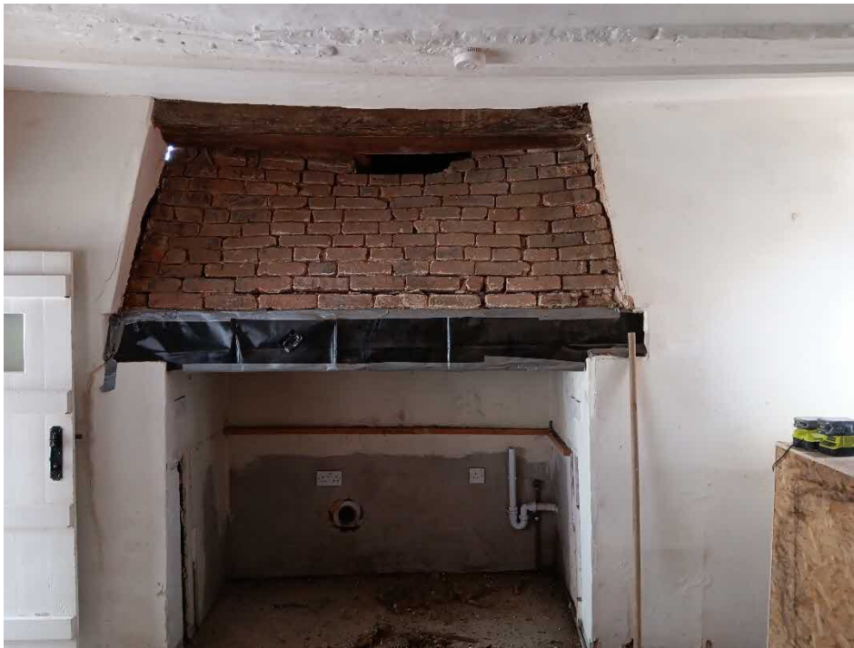
Fig 5: Defective brickwork above fireplace
