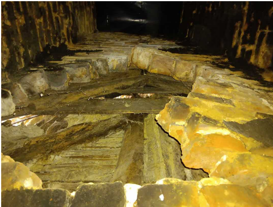
Fig 6: Missing bricks above brick hood below
