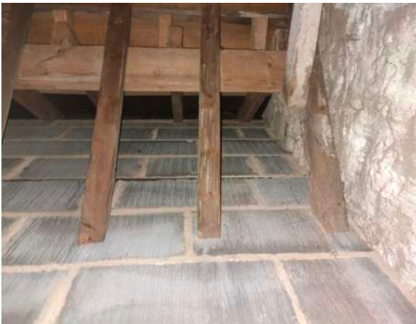
13. The attic space above north room showing block walls and C20 roof structure
