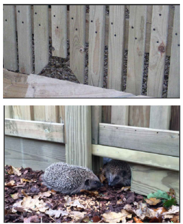
Minimum 170mm dia hole to be cut in the base of Picket & close boarded fencing at a max of every 12metres to allow movement of hedgehogs between gardeners.
