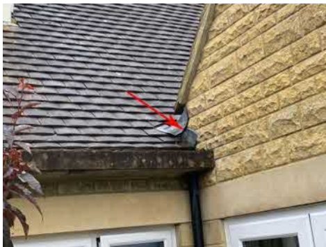
Photo 5: E1 - Red arrow points to gap leading beneath raised lead flashing.
