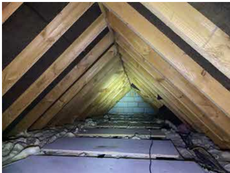
Photo 11: Internal view of loft element showing exposed timbers and bitumen felt underlining. E2
