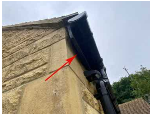
Photo 2: Red arrow points to gaps leading beneath timber fascia board. E2
