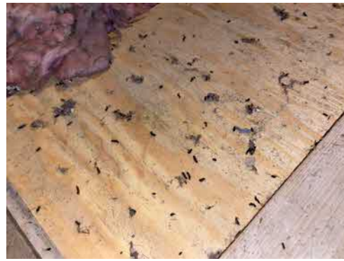
Photo 10: Bat droppings upon floor boards. E1.
