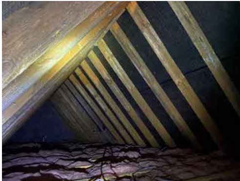
Photo 7: Internal view of loft element showing exposed timbers and bitumen felt underlining. E1
