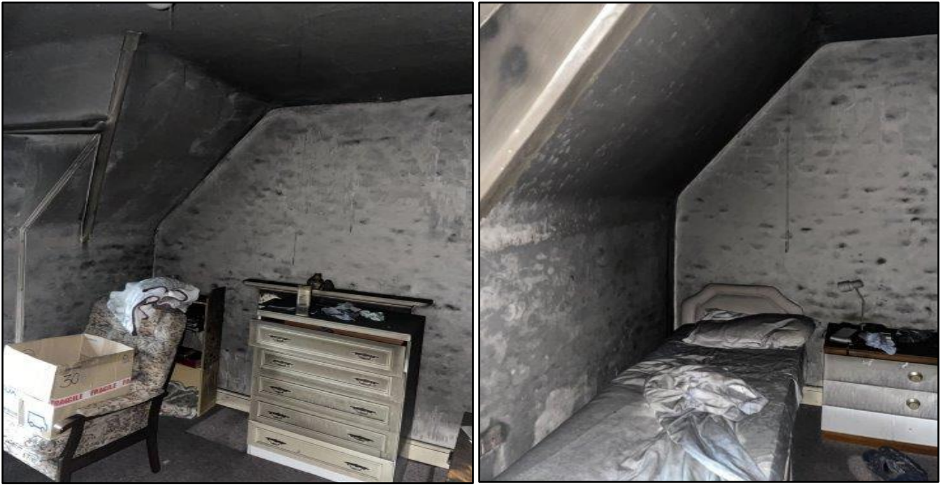
P 5: First Floor – areas of damage (Sedgwick 2024)
