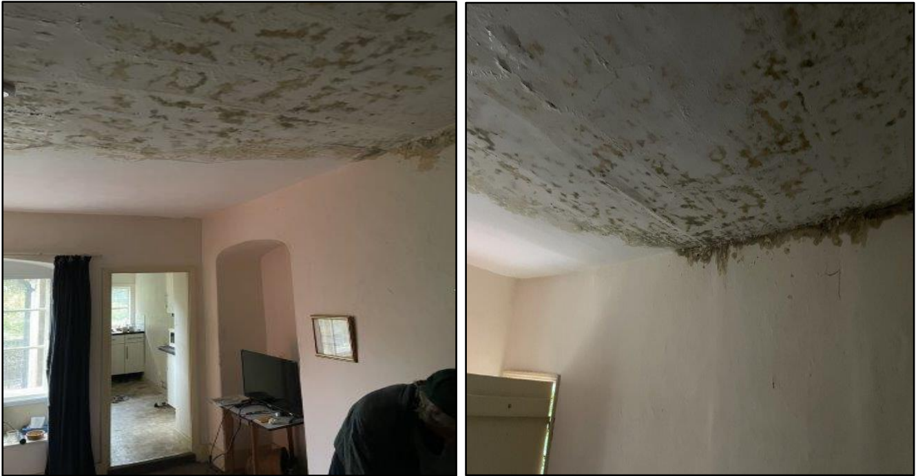
P 1: Ground floor – areas of ceiling damage (Sedgwick 2024)
