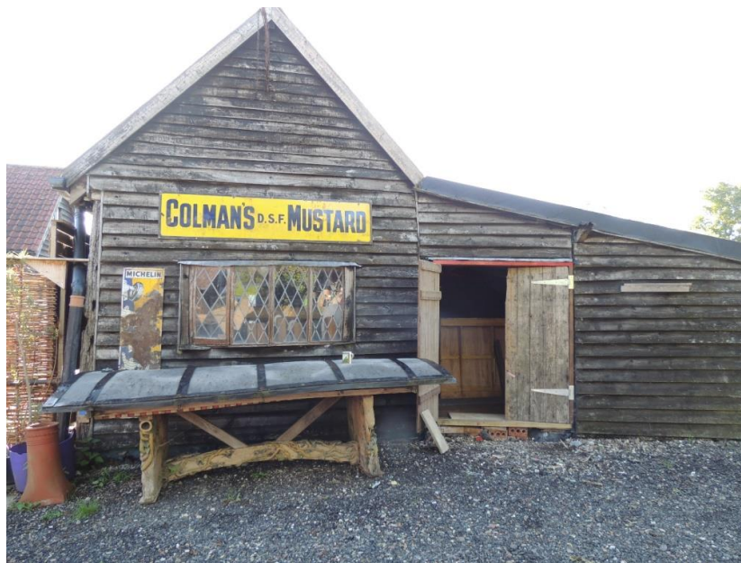
Photo 1: Western elevation. The proposal is to demolish and replace the building with a studio
