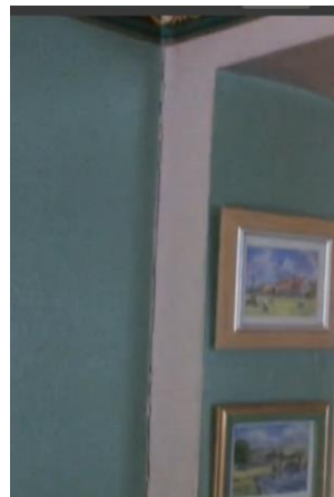
Picture 2: : Internal cracking to rear extension
