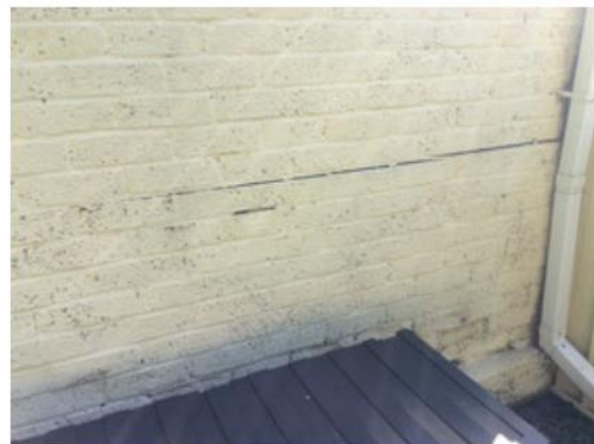
Picture 4: External cracking to garage
