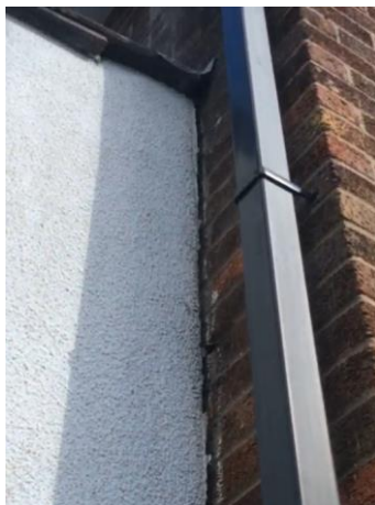
Picture 3: External cracking to rear extension
