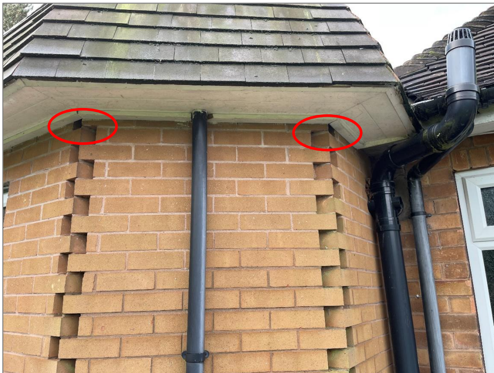
Photograph 4: Gaps in the brickwork (circled red) that could provide bat / bird access into the soffits.
